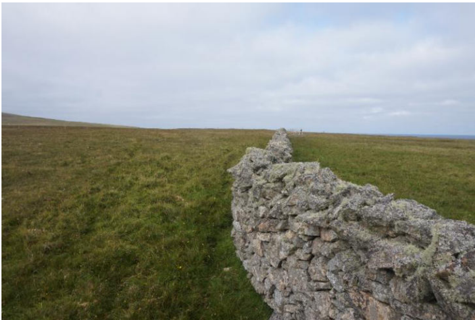
Monitor the bulged section and allow repairs/rebuilding if its condition worsens.
