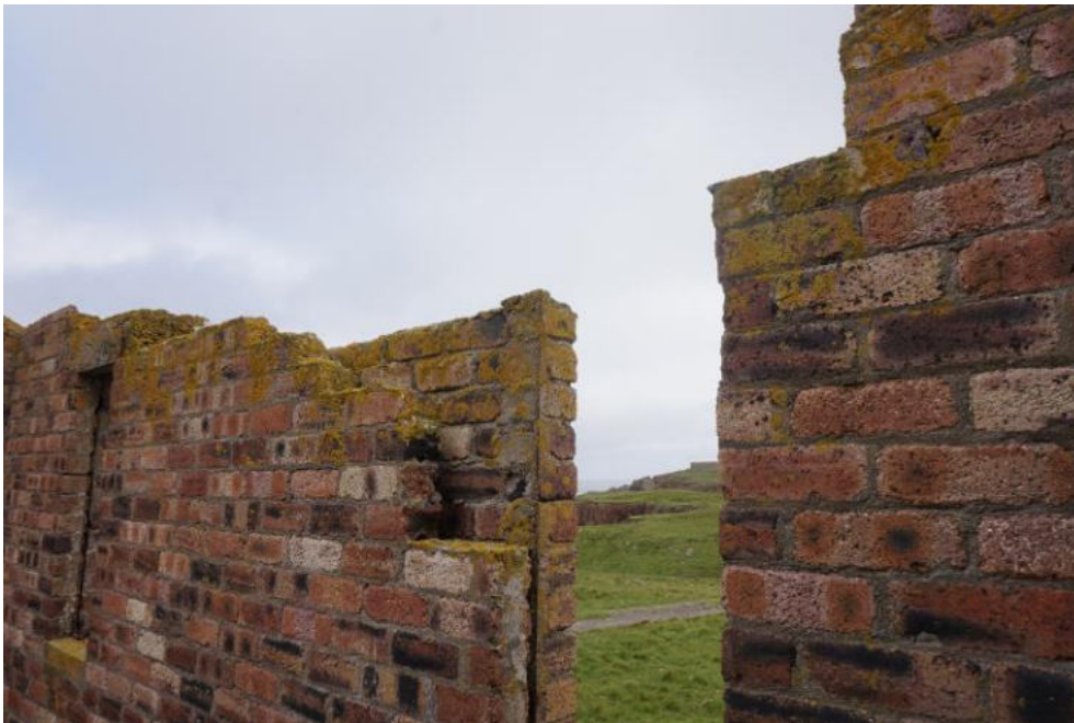
East elevation (internal) with dislodged lintol and fallen wallhead brickwork. To prevent ingress into the cavity, consider resetting the lintol and brickwork to allow the wallhead to be capped in concrete.
