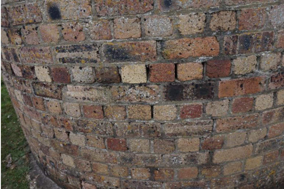
Localised failing wallface joints.
