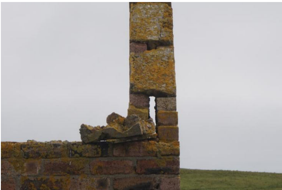
Damaged and dislodged concrete capping to south gable should be removed to reduce health and safety risk. Note that no wall ties are visible within the cavity. Reinstating the wallhead capping will prevent water ingress into the cavity.
