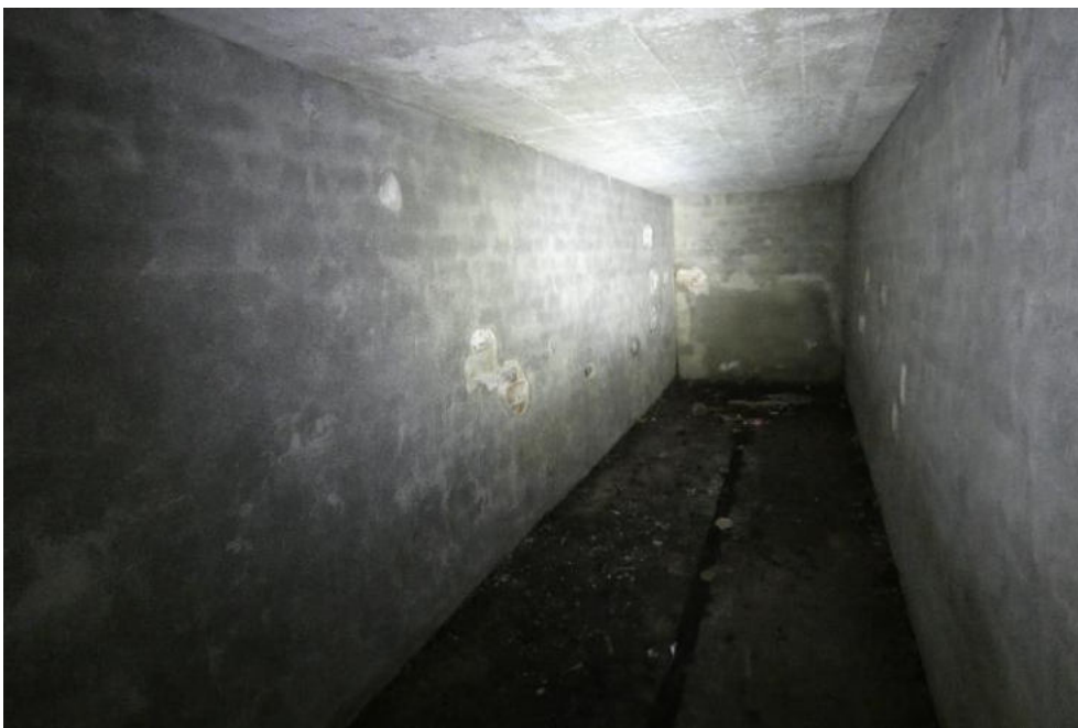
Localised failing render internally.
