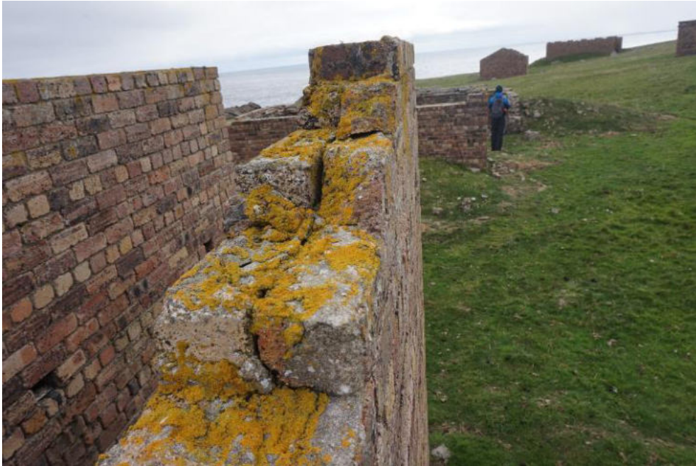
Failing skyward facing joints should be repointed.
