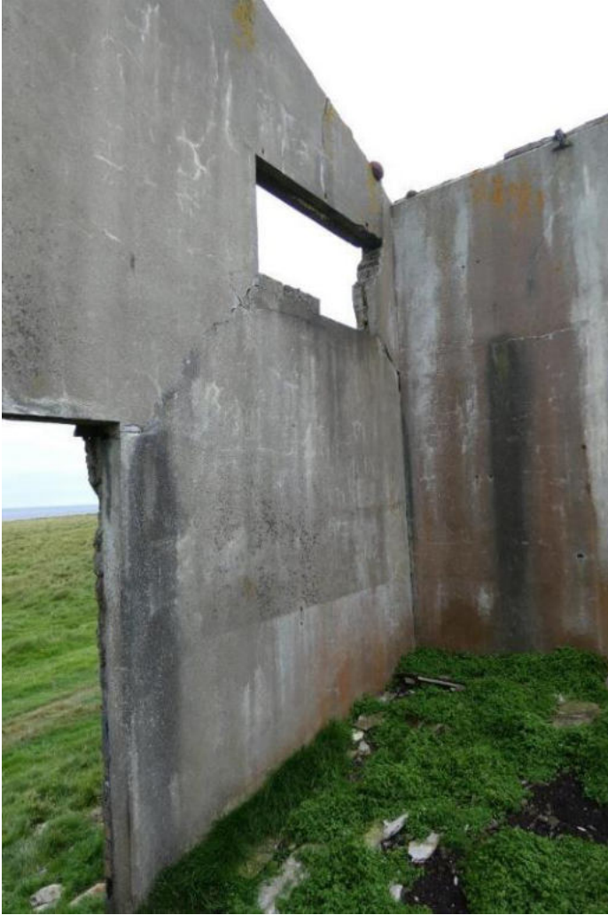
Internal view of east gable. Note how the cracking is right through the masonry.
