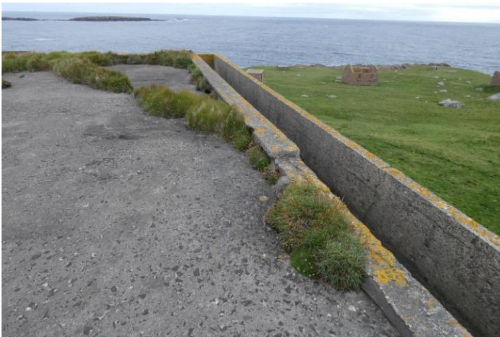
The roofscape. Note missing copes from parapet.
