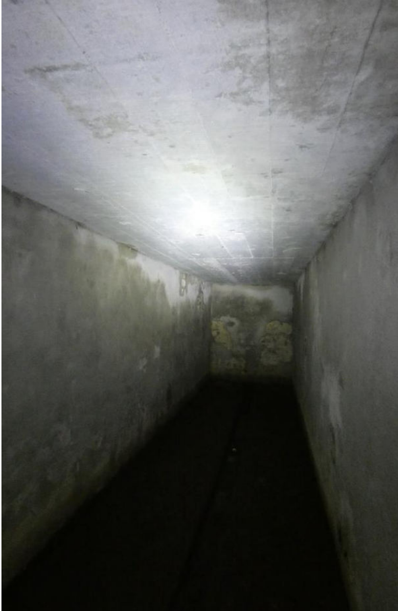
Localised failing render internally.
