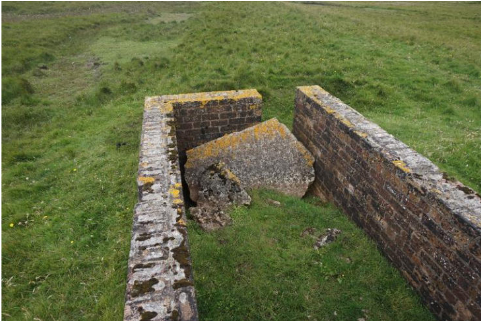
Internal ground levels have increased due to accumulations of soil, and fallen brickwork and concrete.
