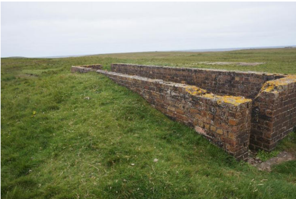
Despite localised failing mortar joints, and damaged and missing brickwork, the structure is in a stable condition.
