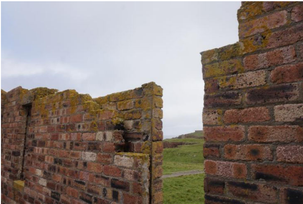
East elevation (internal) with dislodged lintel and fallen wallhead brickwork. To prevent ingress into the cavity, consider resetting the lintel and brickwork to allow the wallhead to be capped in concrete.
