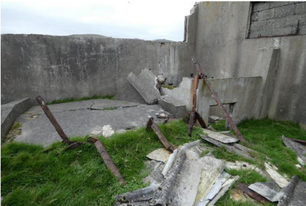
Inside of the west gable. The collapsed upper section can be seen on the floor.
