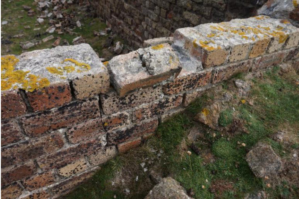
Defective skyward facing joints should be repointed, with allowance for resetting loose brickwork.
