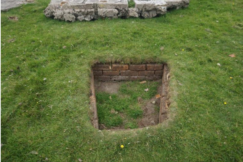
Open joints and loose brickwork to wallheads of brick drainage chamber.
