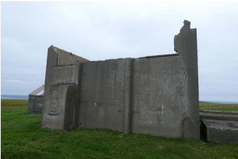
West elevation. The triangular gable has collapsed, falling inwards. Note the full-height crack to the south corner: there is no continuity between the west or south walls – they are free-standing elements.
