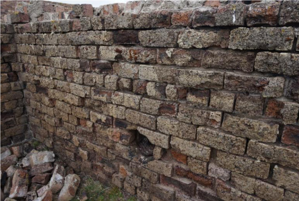
The internal faces are badly fire damaged, requiring extensive consolidation including repointing, resetting loose bricks and replacing badly damaged bricks.
