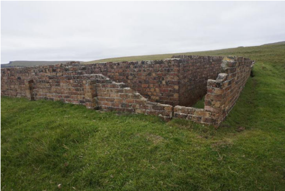
Structural issues in the northeast corner. Vertical cracks on the east elevation of the inner and out skins and a pronounced lean to the north wall of the outer skin. Cracks should be repointed and monitored to assess ongoing movement. The leaning outer skin should either be made safe by extending the earth banking eastwards to prevent further outward rotation or taken down to a safe height. The external wall generally does not have inherent stability generally. This issue should be addressed if increased footfall is expected.
