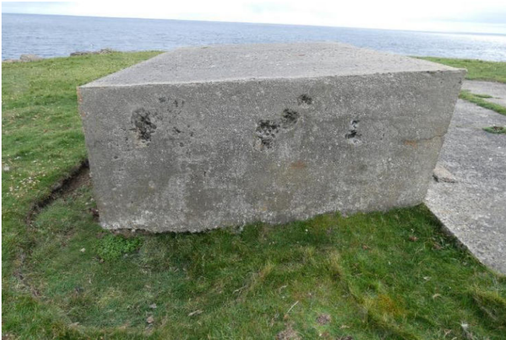
Localised spalling and damage to external walls.
