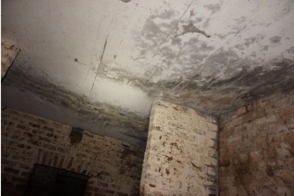
Damp staining and discolouration to underside of concrete roof slab.
