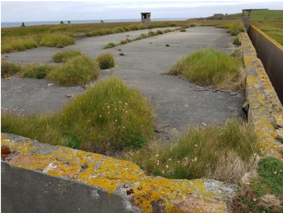
Looking across the roofscape. Note cracked asphalt, vegetation and missing concrete copes from wallheads.
