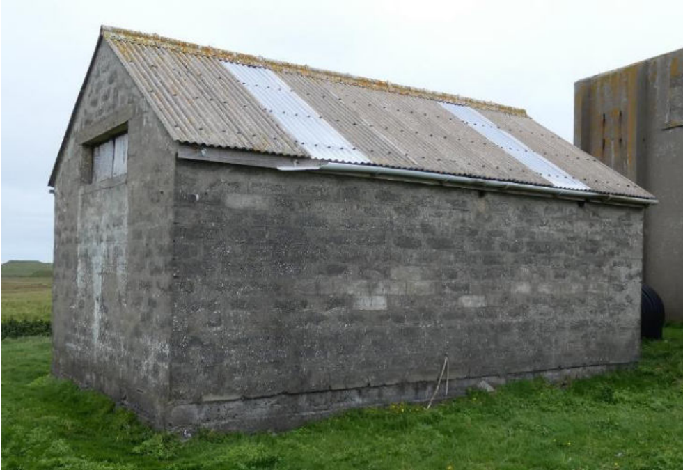
West elevation: Replace rainwater goods. Decorate facia.
