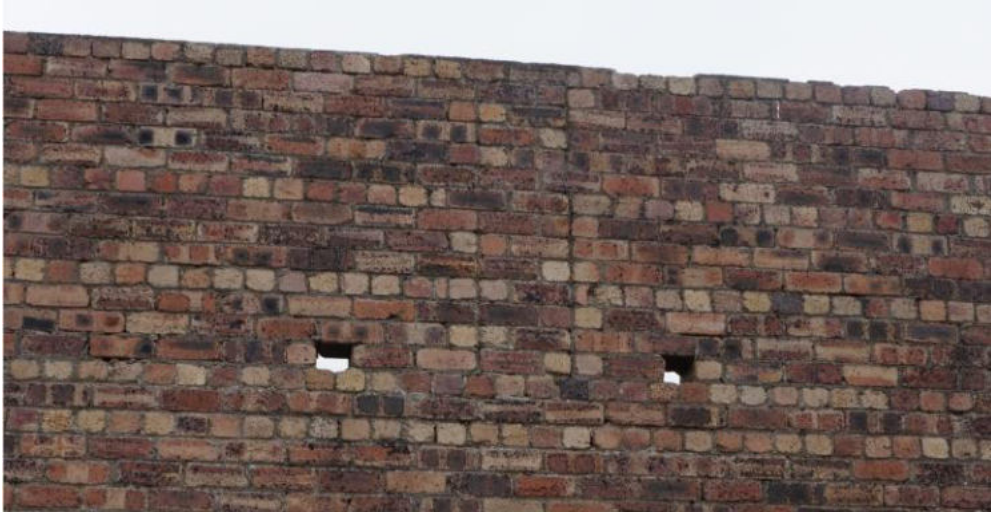
Cracks at higher levels are aligned with the upper piers which are poorly tied to the adjacent thinner single brick thick infilled brickwork.
