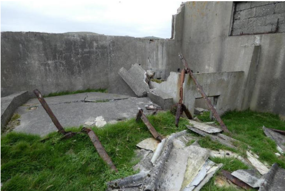
Inside of the west gable. The collapsed upper section can be seen on the floor.
