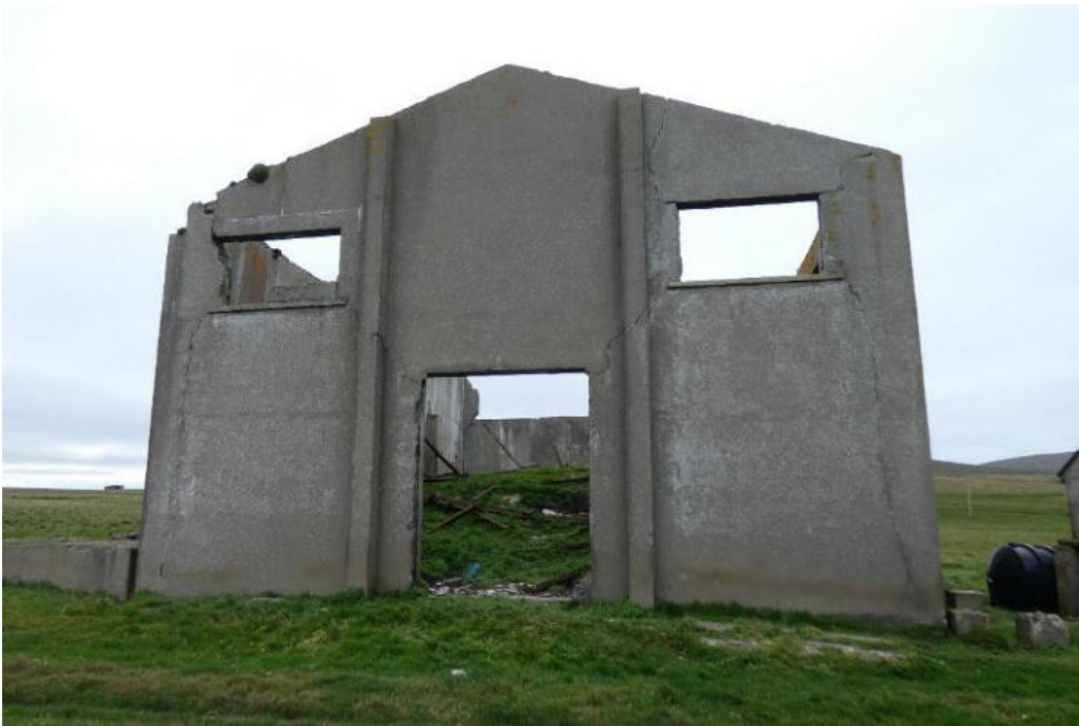
East elevation. Note the vertical cracking at each corner. Note the diagonal cracking between the entrance opening and both window openings and how this cracking continues up to wallhead: this elevation is a stack of independent, thin, tall, wall panels sitting atop each other.
