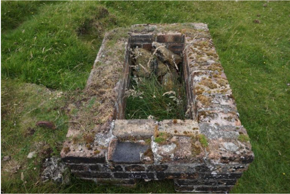
Failing joints to wallhead supporting vegetation growth. Localised damaged bricks.
