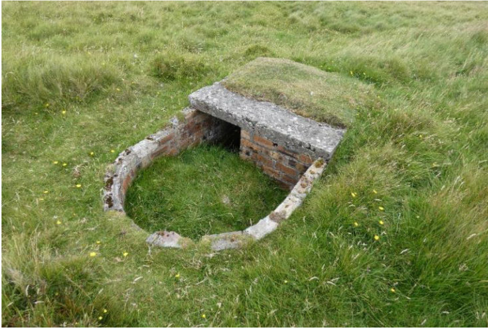
General view. Note damaged wallhead bricks.
