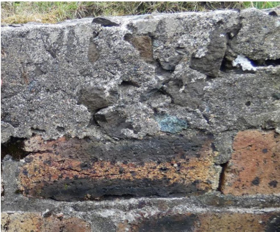
Defective brick joints and exposed aggregate to roof slab.
