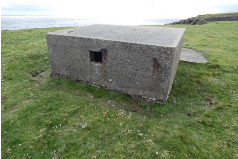
Localised cracking and rust staining.
