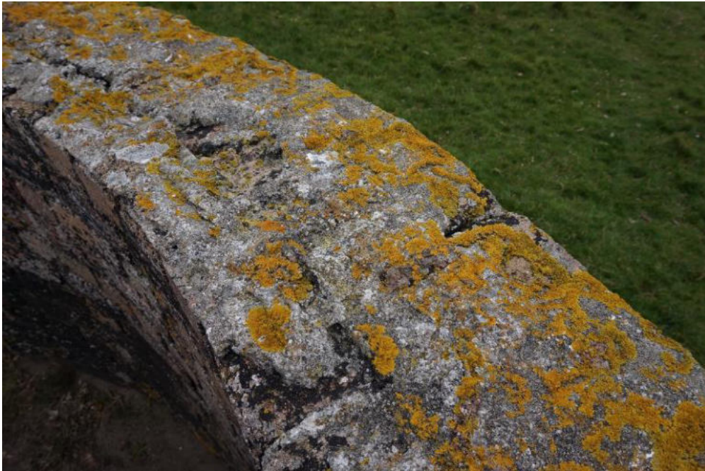
Localised failing skyward facing wallhead joints.
