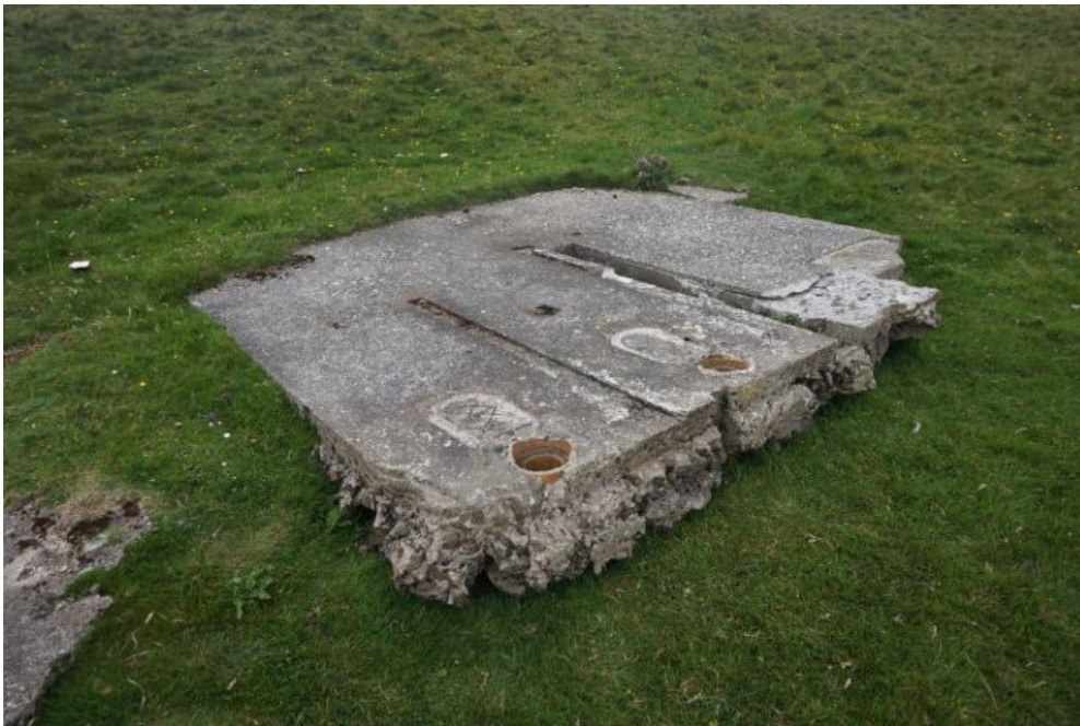
East concrete base with spalling upper face.
