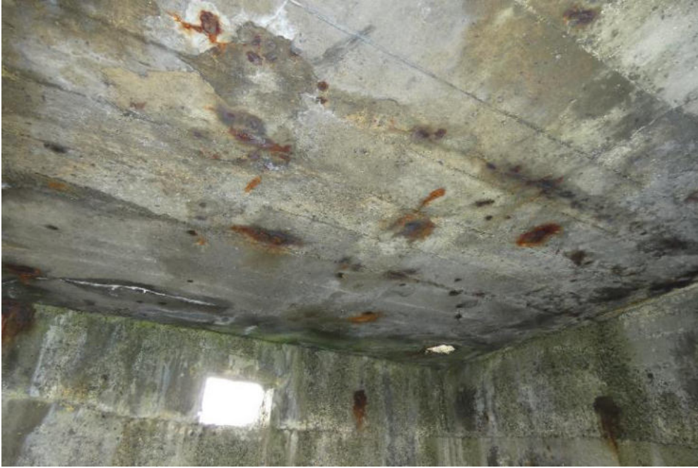
Hairline cracking, rust staining, leaching and discolouration to the soffit of the roof structure.
