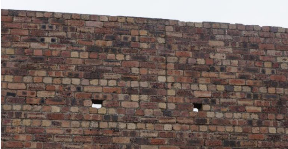
Cracks at higher levels are aligned with the upper piers which are poorly tied to the adjacent thinner single brick thick infilled brickwork.
