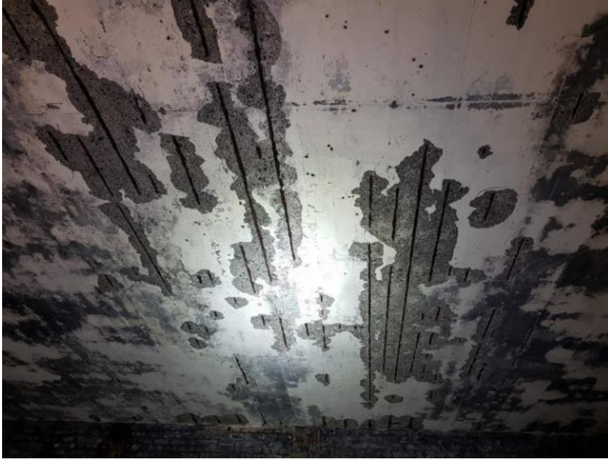
General loss of concrete from the internal soffit of the roof slab.
