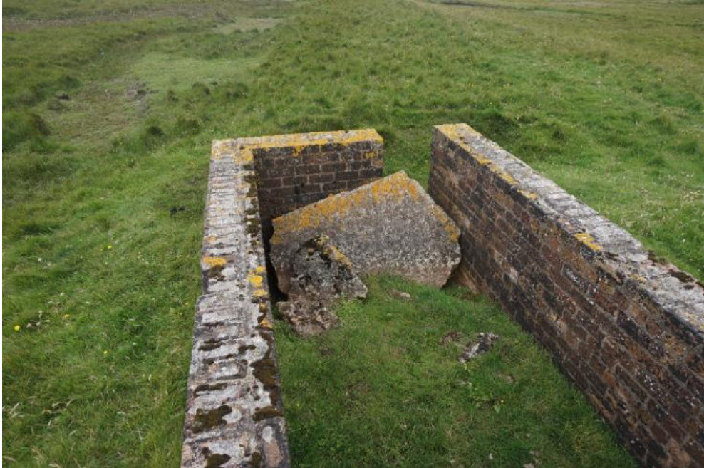
Internal ground levels have increased due to accumulations of soil, and fallen brickwork and concrete.
