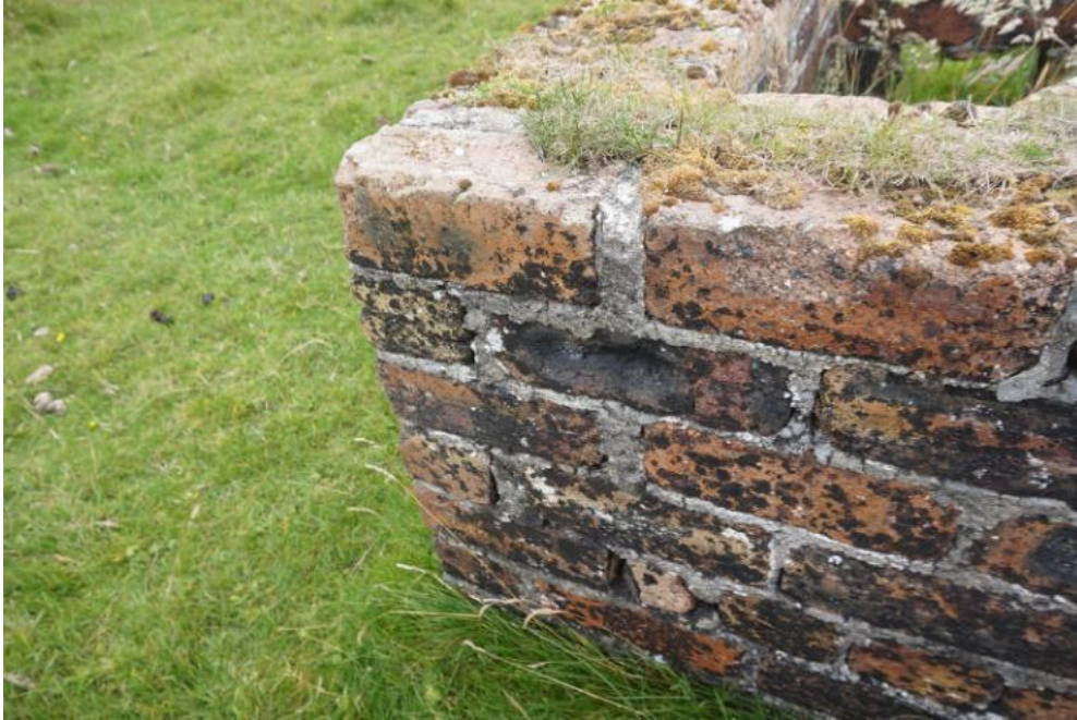
Failing joints to wallhead supporting vegetation growth. Localised damaged bricks and open joints to wall face.
