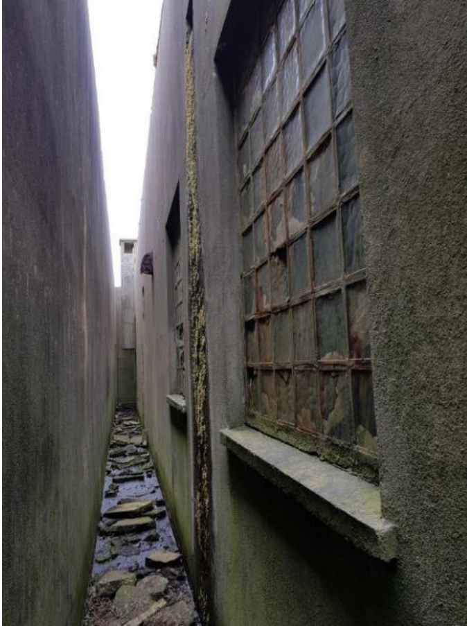
Note debris and build up of water in external perimeter.
