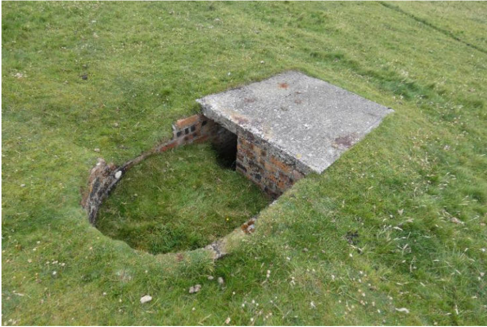
Missing wallhead brick work and defective mortar joints. Minor concrete spalling at slab edge.
