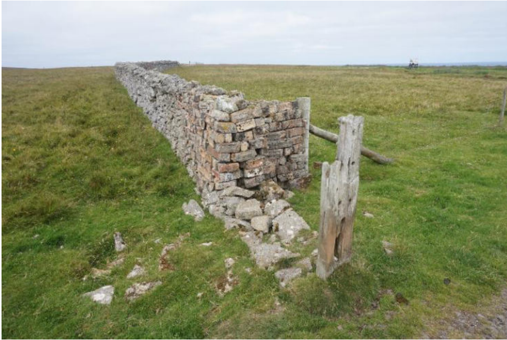
General view north: Brick repairs immediately north of the access road. The repairs remain functional. Rotten timber gate post.
