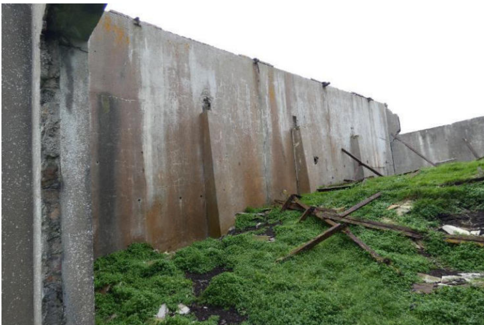
The internal piers do not appear to be fully or properly bonded to the masonry of the external walls.
