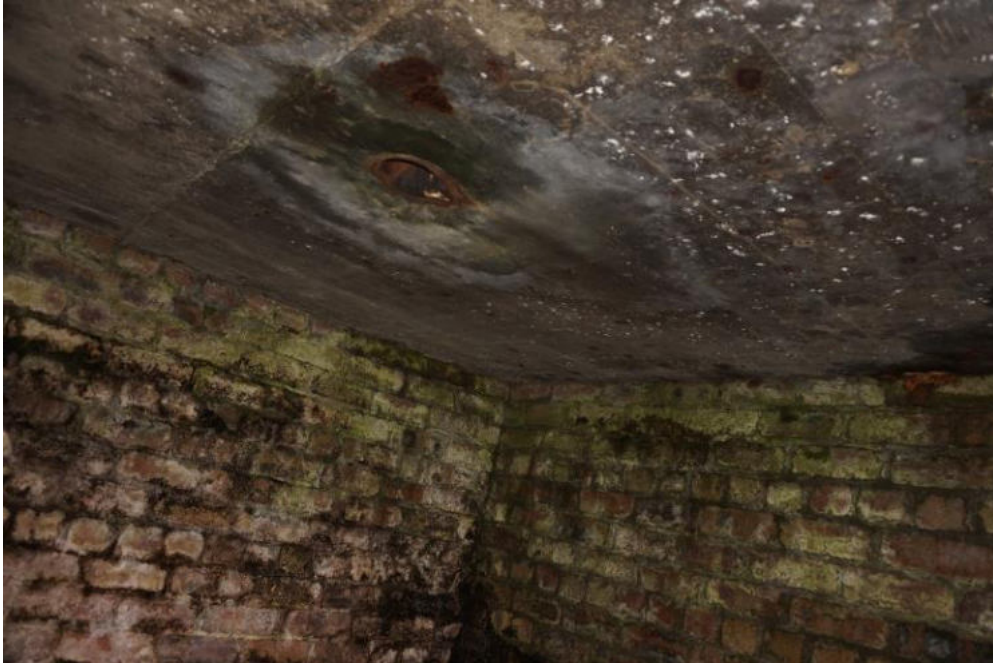
The vent pipe is blocked from above by soil and grass. Localised rust staining was observed on the soffit of the roof slab. No obvious spalling of the concrete.
