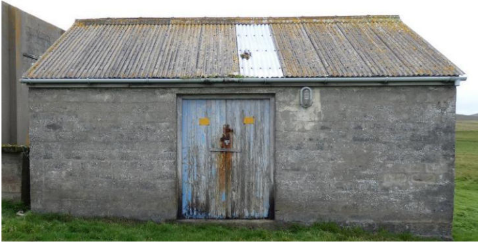
East elevation: Replace rainwater goods. Joinery repairs to doors prior to full joinery redecoration.
