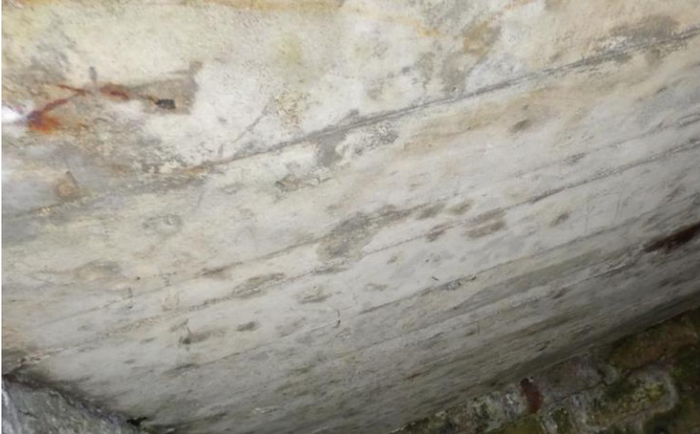
Minor spalling and exposed reinforcement.
