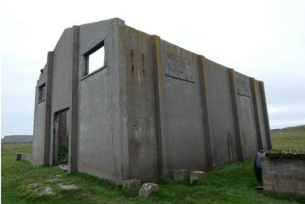
The northeast corner of the building. Note the vertical crack in the east elevation at the corner: there is no continuity between the west or south walls – they are free-standing elements.
