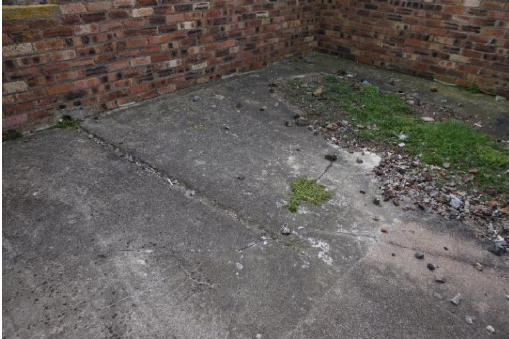
Cracked concrete floor slab supporting vegetation growth.
