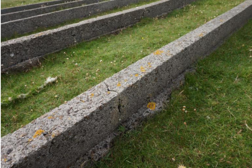
Despite widespread cracking, the walls remain stable.
