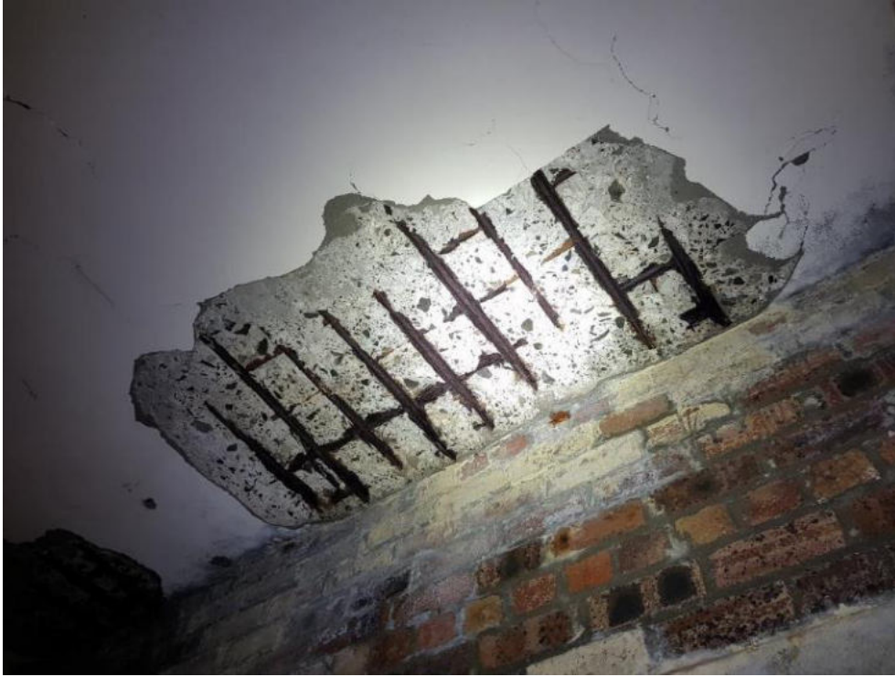
Spalling concrete caused by expansive corrosion of reinforcement.
