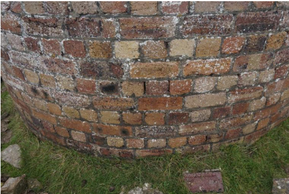
Localised failing joints to wall face.
