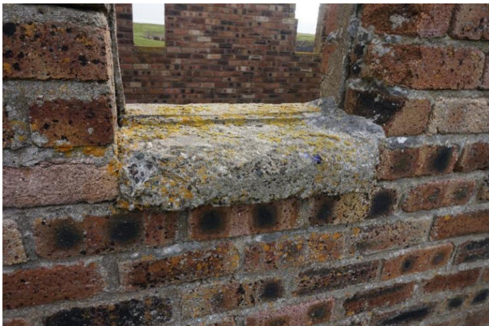
Disaggregating concrete cill.
