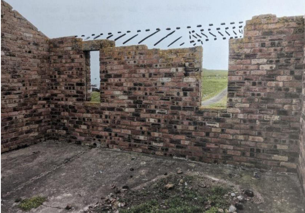
Fig. 12: To minimise water ingress into the cavity wall of the Guard Hut, and the displaced lintel and brickwork could be reinstated to wallhead level to allow capping like that originally placed over the gable wallheads. This work would reduce the rate at which the cavity wall ties will deteriorate.
