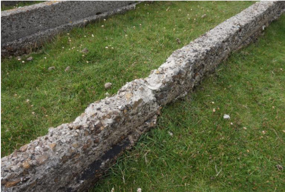
Localised spalling and disaggregation at the eastern end of one of the centre sleeper walls.
