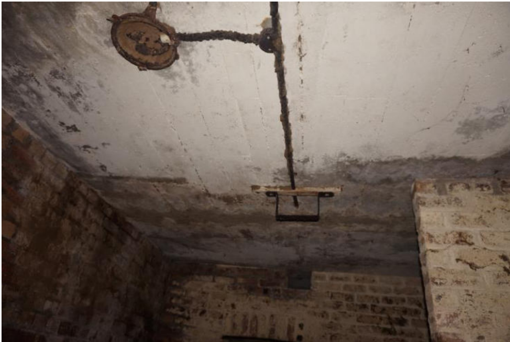
Corroded surface mounted servicing.
