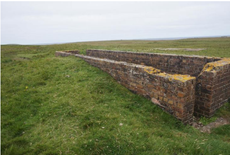
Despite localised failing mortar joints, and damaged and missing brickwork, the structure is in a stable condition.
