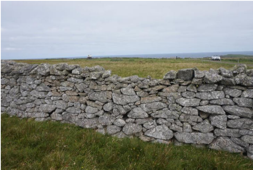
Displaced cope stones should be reinstated.
