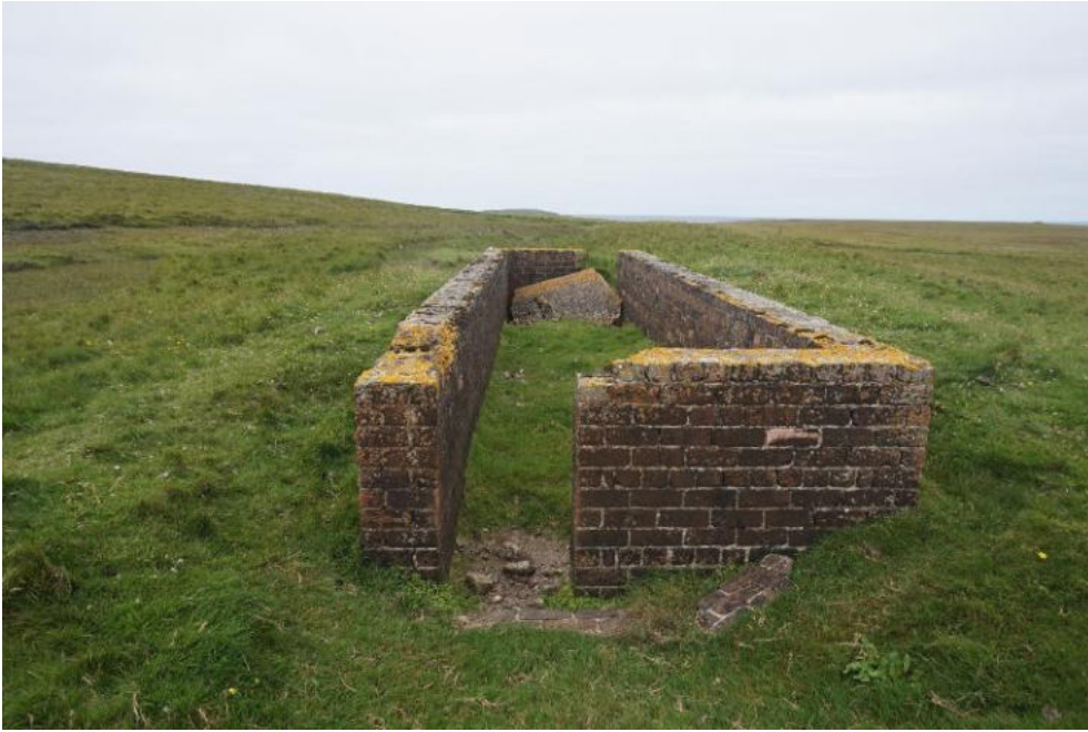
View from south showing missing wallhead brickwork, and displaced bricks and concrete roof slab.
