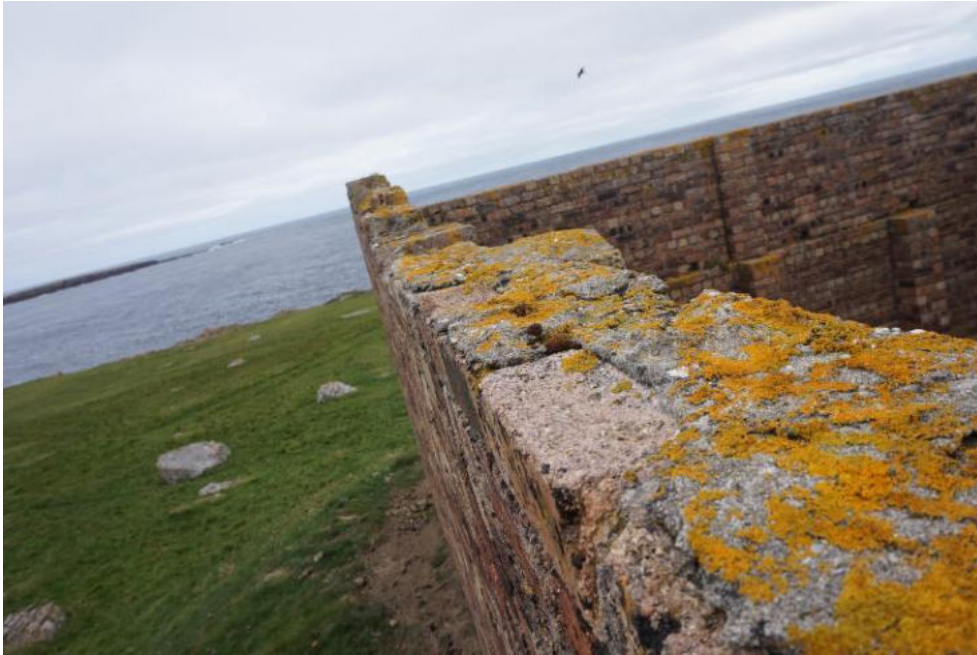
Failing skyward facing joints should be repointed, with allowance for rebedding loose bricks.
