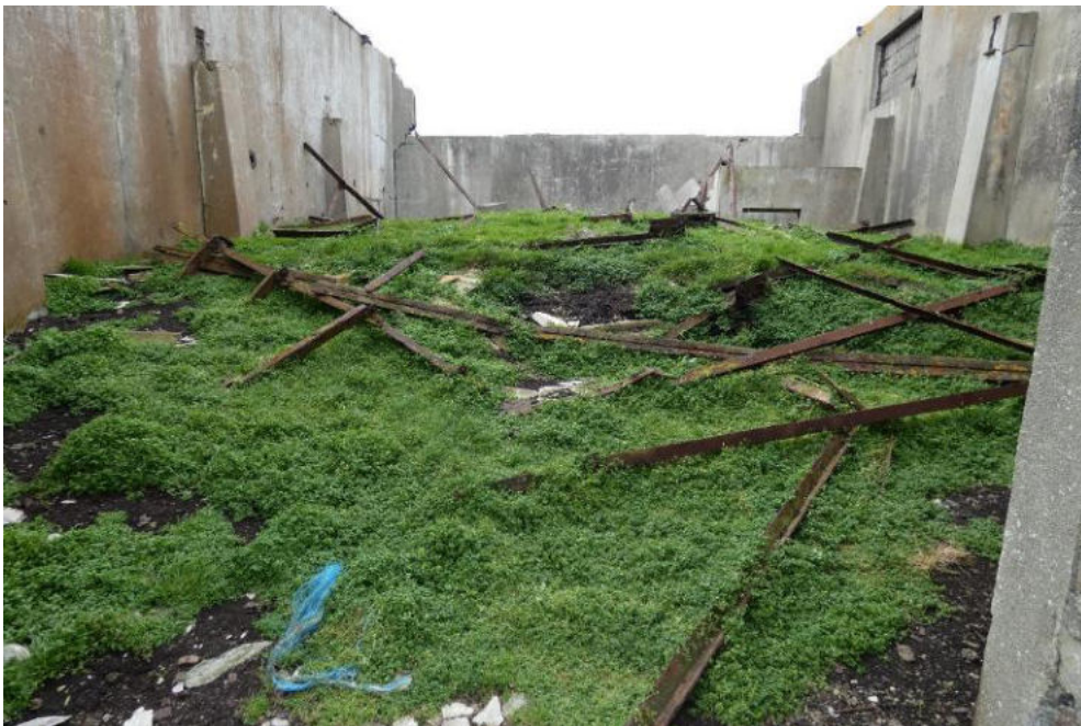
Inside the building. Note remains of the roof structure and asbestos roof tiles.
