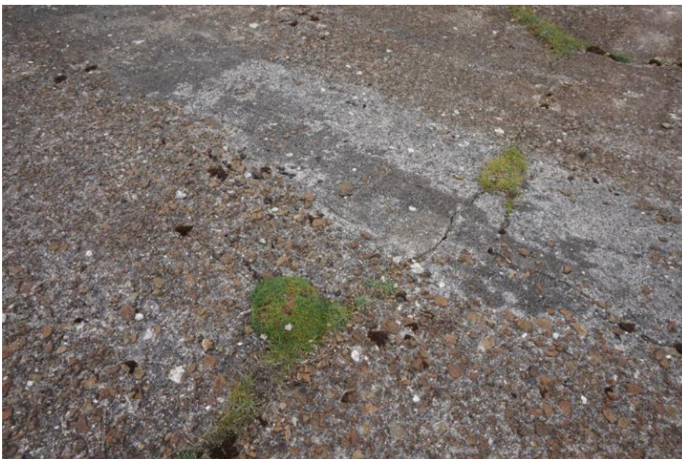
Cracked and disaggregated floor slab supporting vegetation growth.
