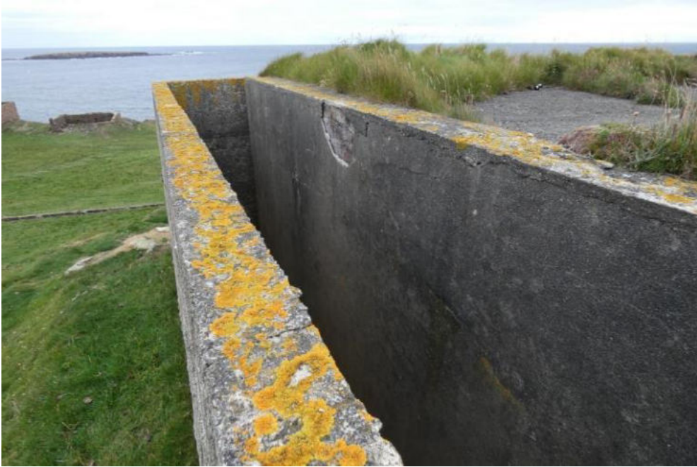
As before. Note the loss of render from the wall of the building.
