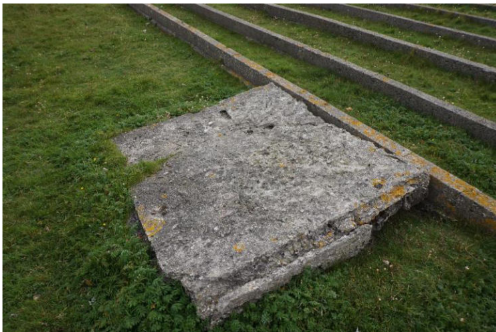
The entrance platt remains stable despite misalignment and localised cracking, spalling and disaggregation.
