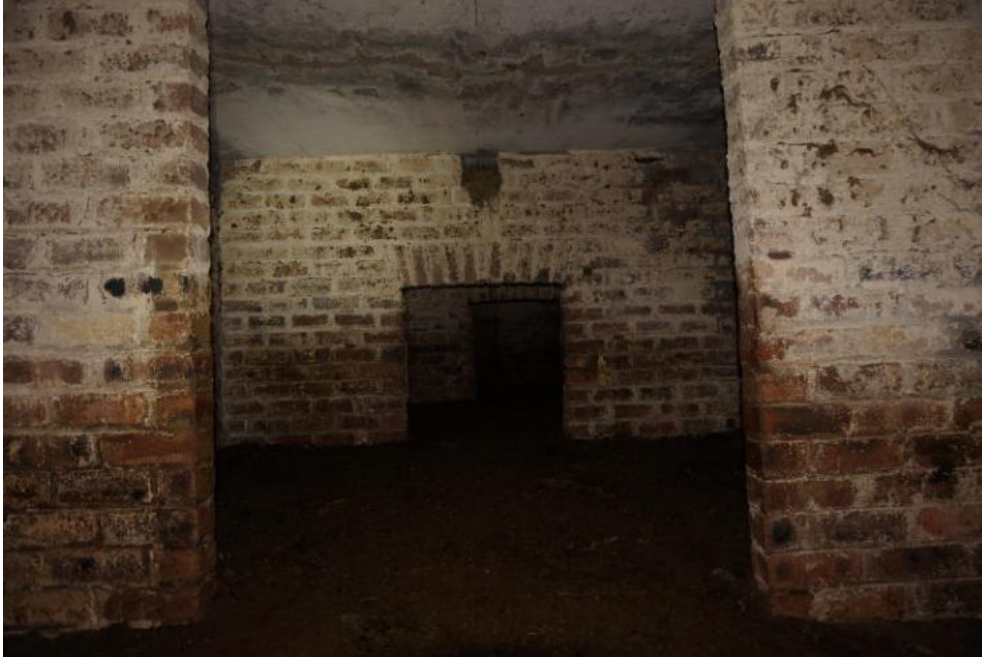
Internal painted surfaces and damp stained and affected by salts from the large accumulations of animal faeces.
