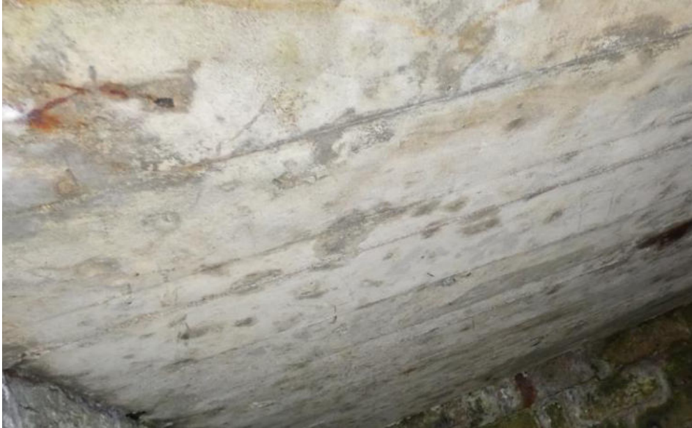
Minor spalling and exposed reinforcement.
