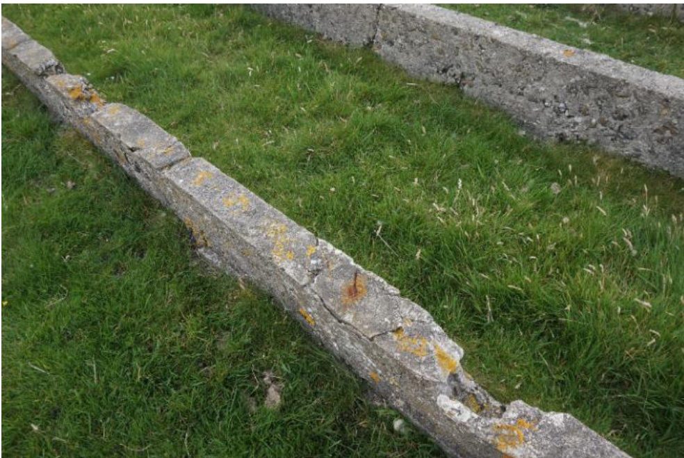
Localised spalling where corroded wallplate fixings survive.
