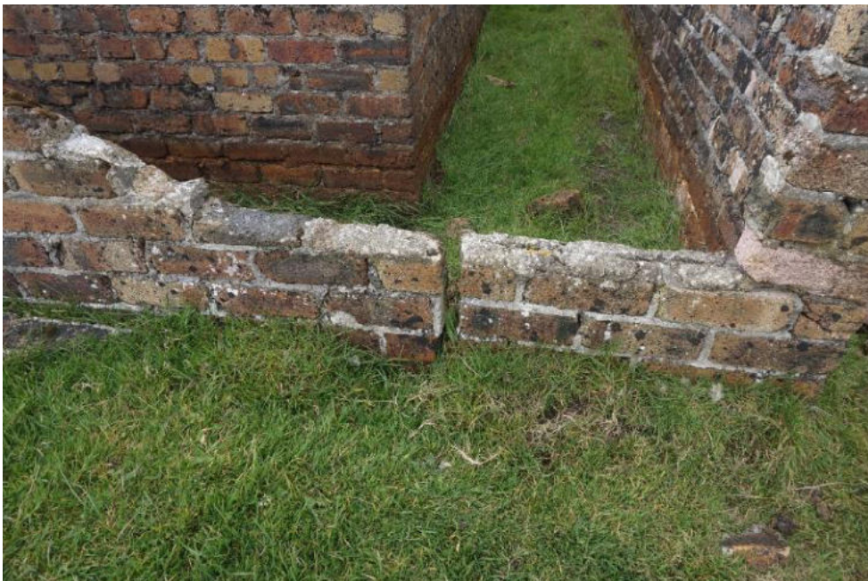
Cracked brickwork to the east facing half brick thick outer skin adjacent to the leaning north wall.
