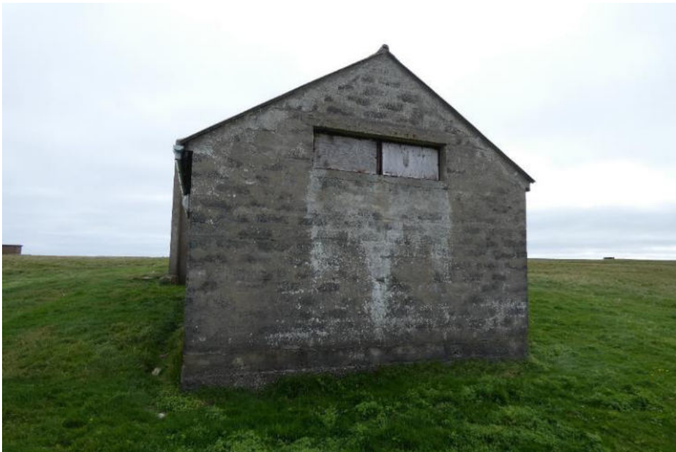
North elevation: Repoint cracked lintol and monitor. Replace boards to window and decorate.
