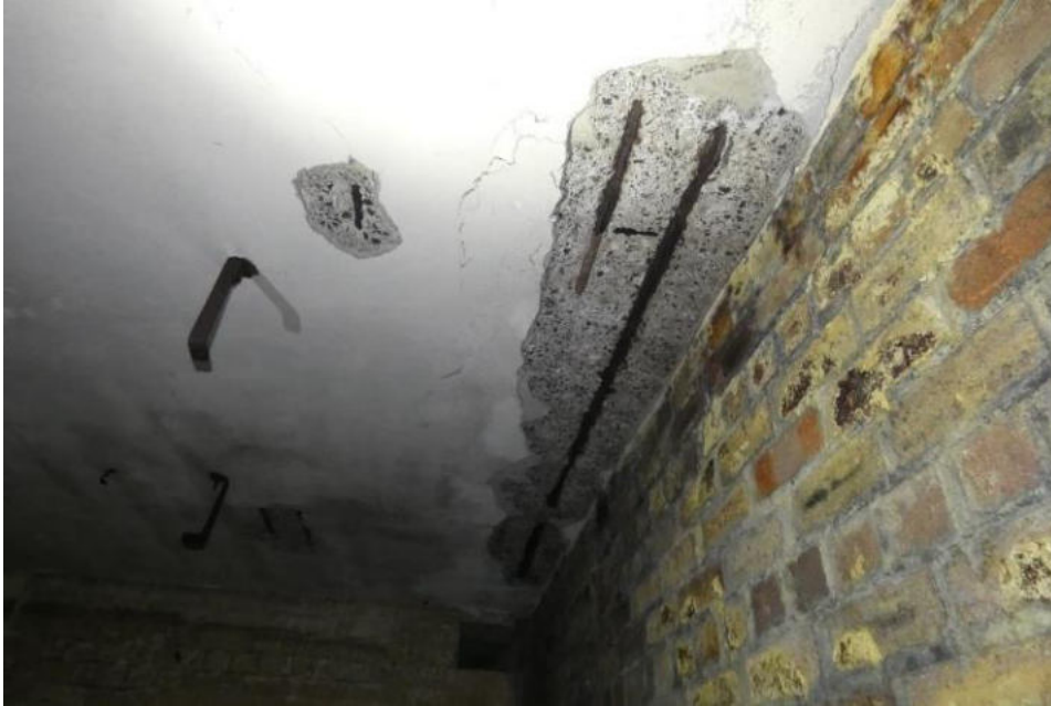
In places, expansive corrosion of reinforcement is causing spalling of concrete from roof soffit.
