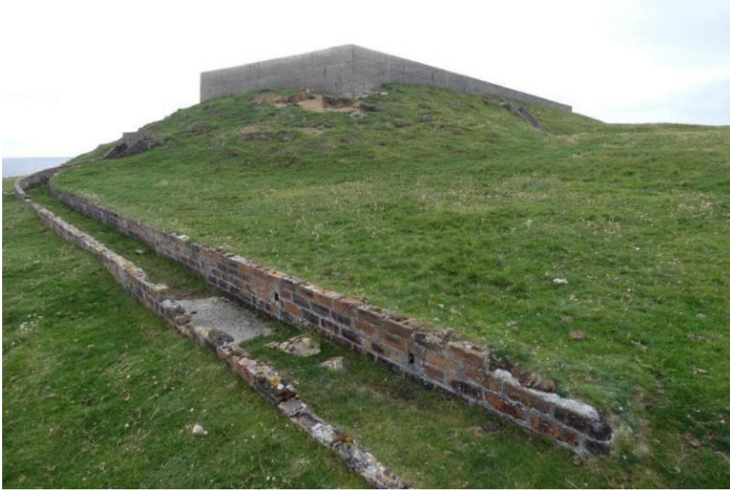
The external brick service trench. Note general deterioration of top courses of its masonry. Note also the loss of material from the embankment about the blast walls.
