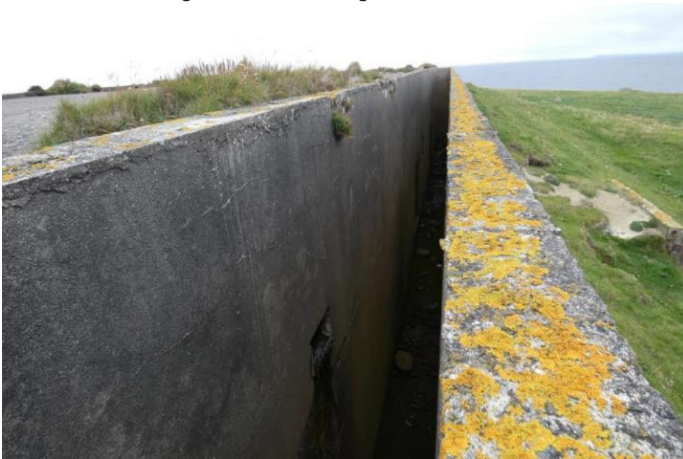
From the top of the embankment looking down into the gap between blast wall and building. The discharge point from the rainwater roof outlet can be seen partway down the wall of the building. vegetation growing from this outlet is blocking it.
