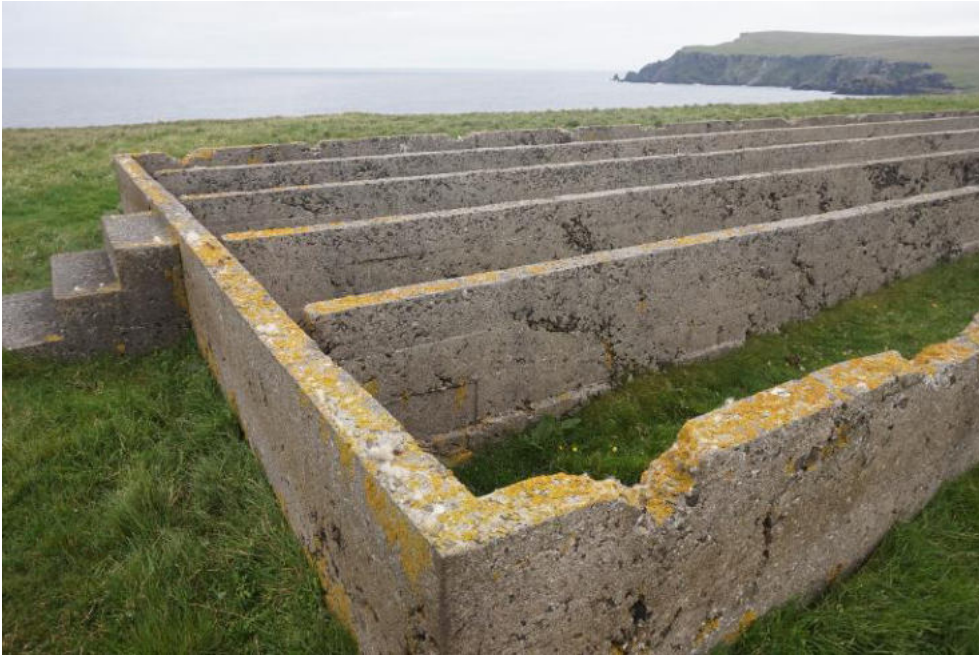
Damaged concrete is limited to the perimeter walls, suggesting it was caused during demolition works and removal of the wallplate fixings or when the fixings corroded at a later date causing localised spalling. Note poorly mixed and compacted concrete.
