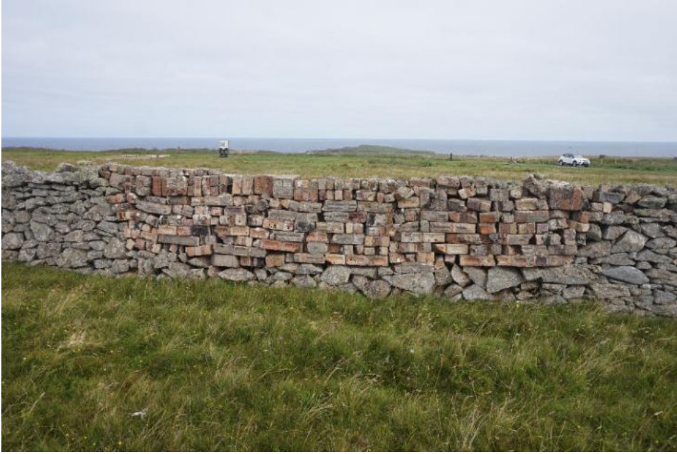
The repair using salvaged bricks c.40m north of the access road remains in good condition.
