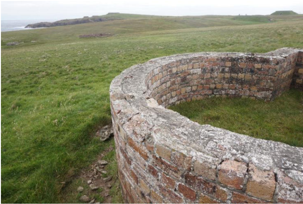
Localised open joints and damaged brickwork to wallhead.
