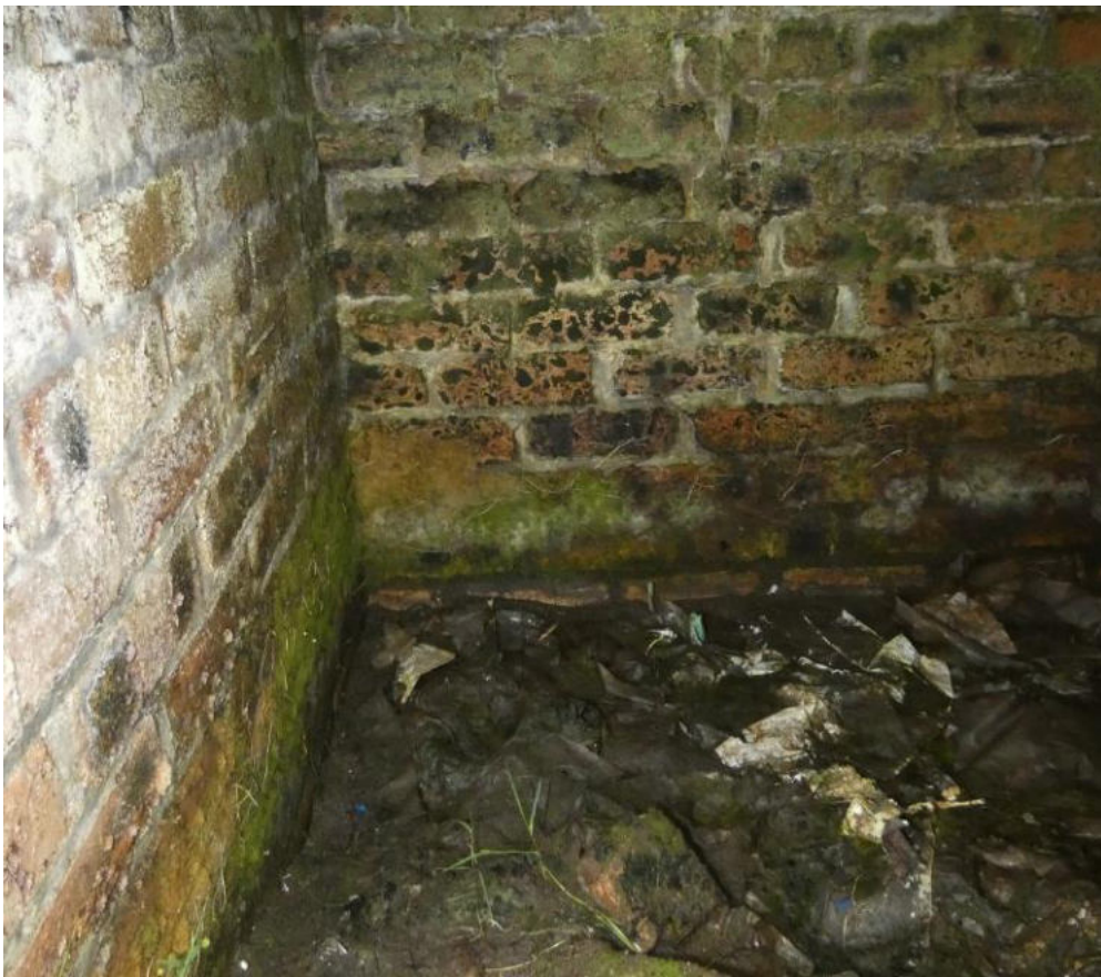
Saturated brickwork below covered area.
