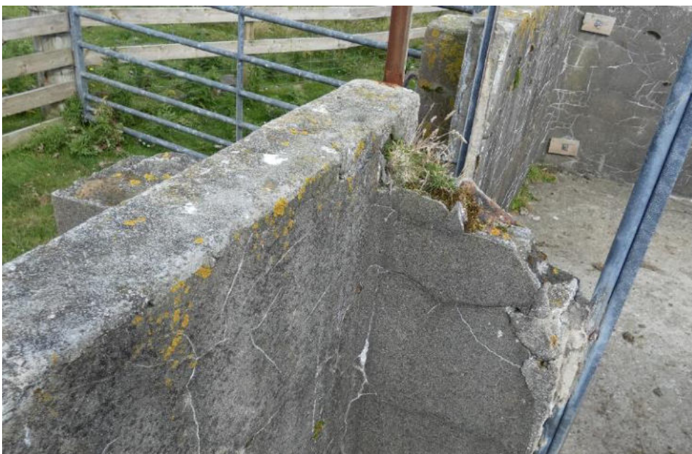
Localised damaged wallhead brickwork.
