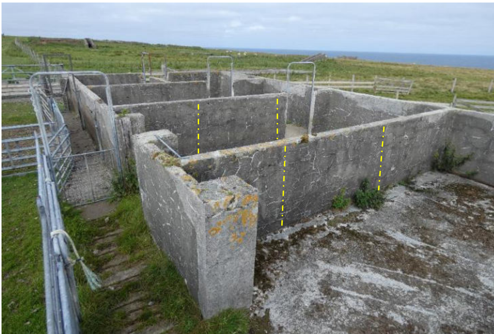
The cement render is extensively cracked and in some areas is supporting vegetation growth. The concrete floor has minor disaggregation and is supporting vegetation growth. The relatively long and slender internal partition walls depend on the integrity of the mortar in their bed joints for their stability. The robustness of these walls can be increased with the introduction of new buttresses at key points (indicated)
