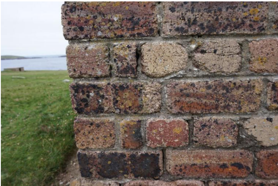
Localised filling wall face joints and minor cracking should be repointed.
