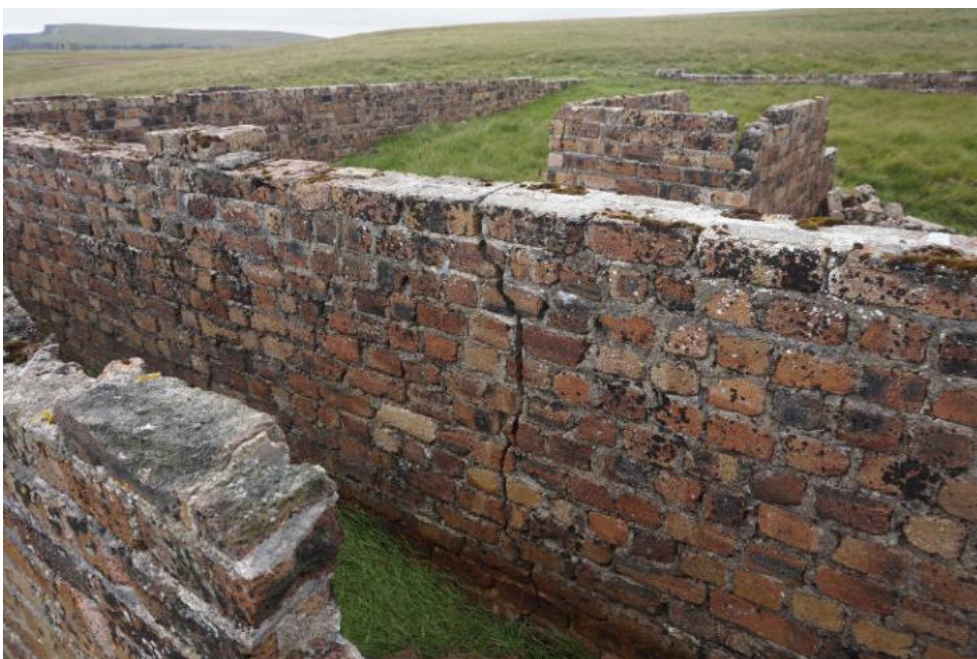
Cracked brickwork to the single brick thick east facing inner skin. Cracks should be repointed to allow future monitoring.
