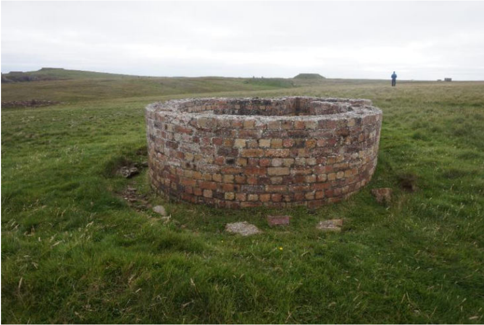
General view from south showing damaged wallhead brickwork and localised failing joints to wall face. Displaced bricks around base of wall.
