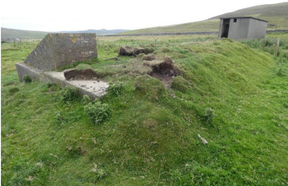
Replacing the missing and damaged earth and turf banking will protect the structure below.
