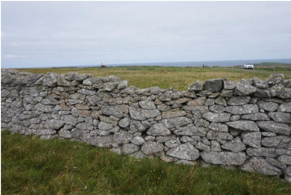
Displaced cope stones should be reinstated.
