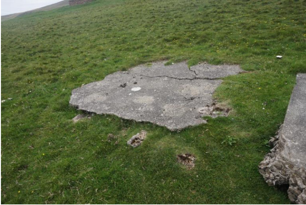
West concrete base has subsided resulting in extensive cracking.
