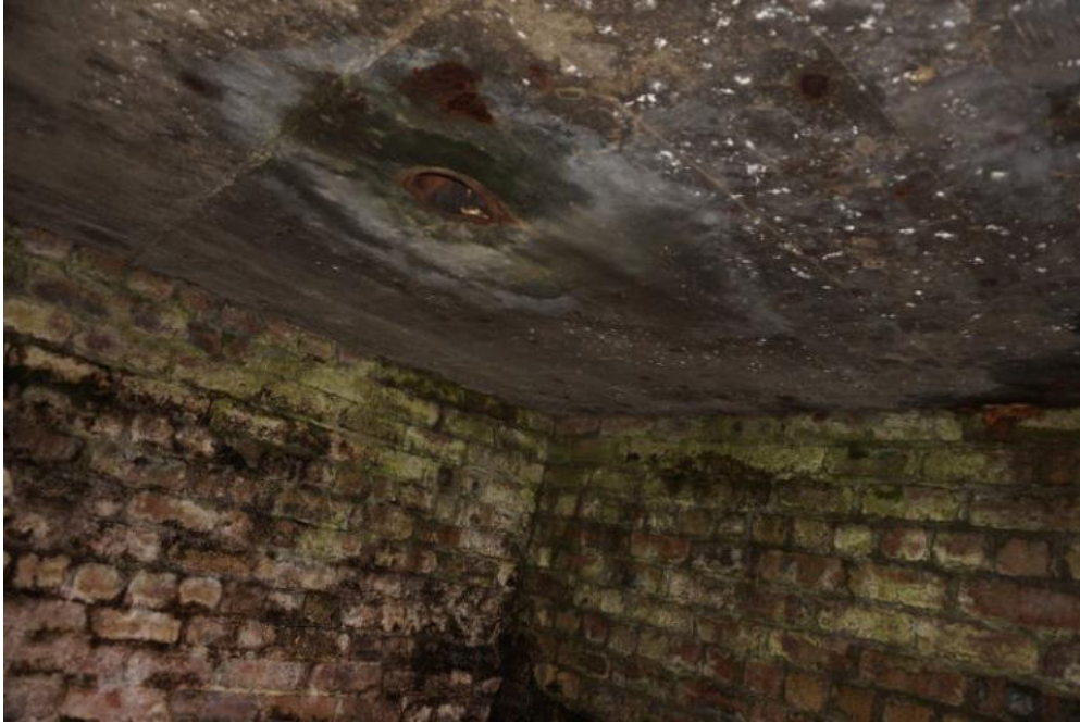
The vent pipe is blocked from above by soil and grass. Localised rust staining was observed on the soffit of the roof slab. No obvious spalling of the concrete.
