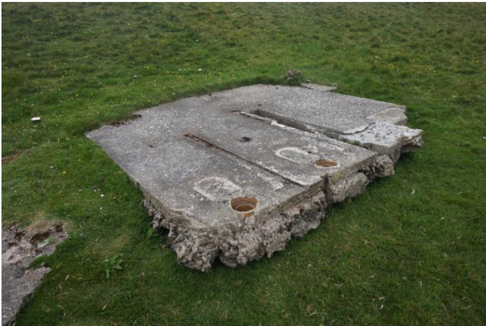
East concrete base with spalling upper face.
