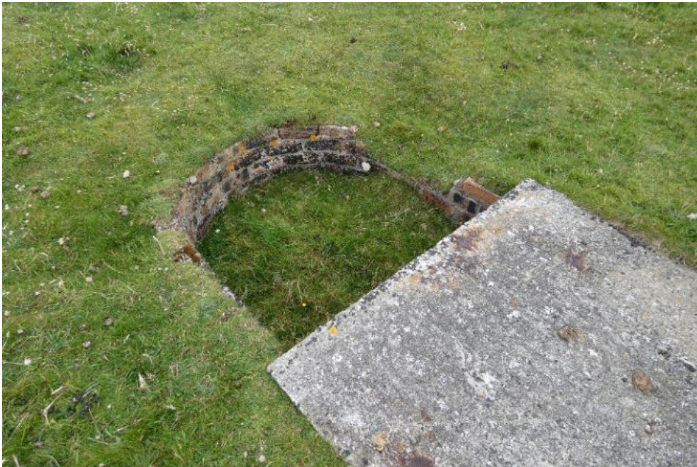
Missing wallhead brick work and defective mortar joints. Localised rust staining to concrete roof slab.
