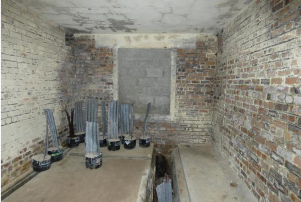
As 10. Note cracked ceiling plaster and indications of general dampness in the brick masonry.
