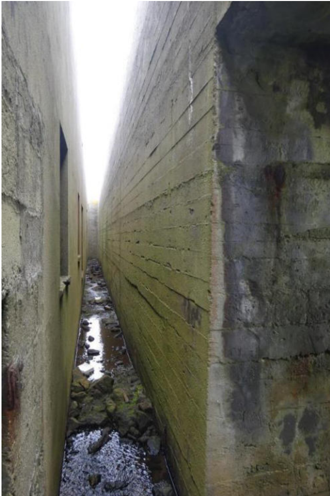
Looking between the blast walls and building proper. Note build up of debris and water.
