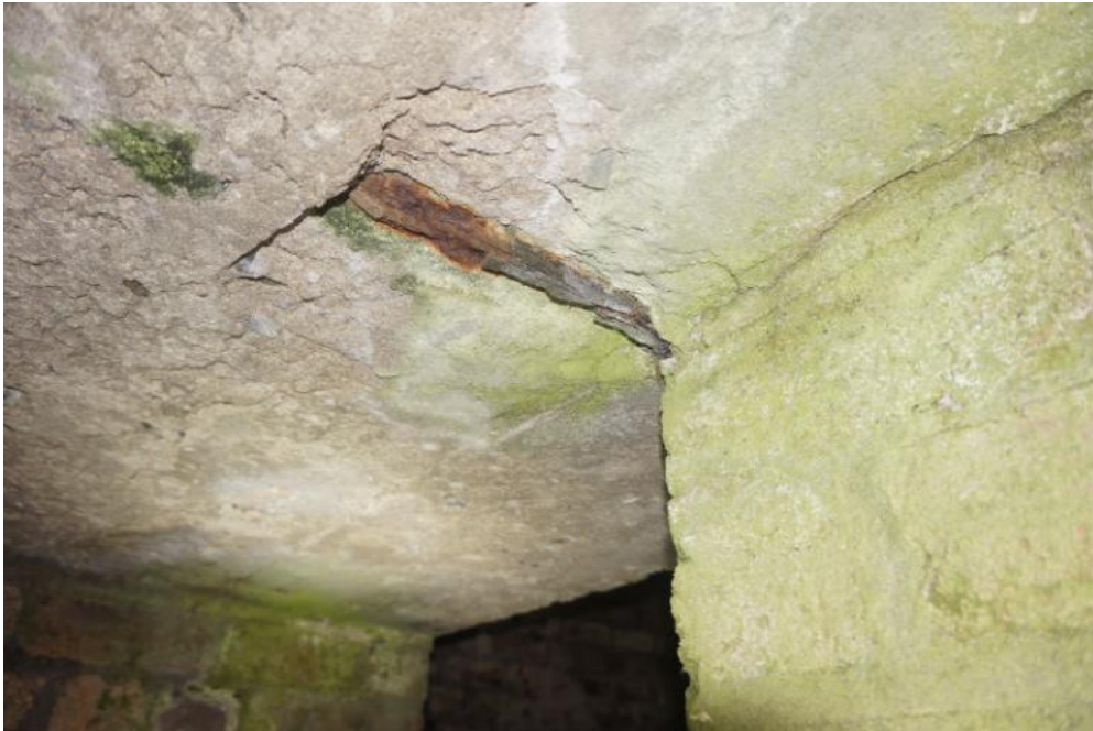
Despite the lack of roof finishes, only minor corrosion of reinforcement was observed.
