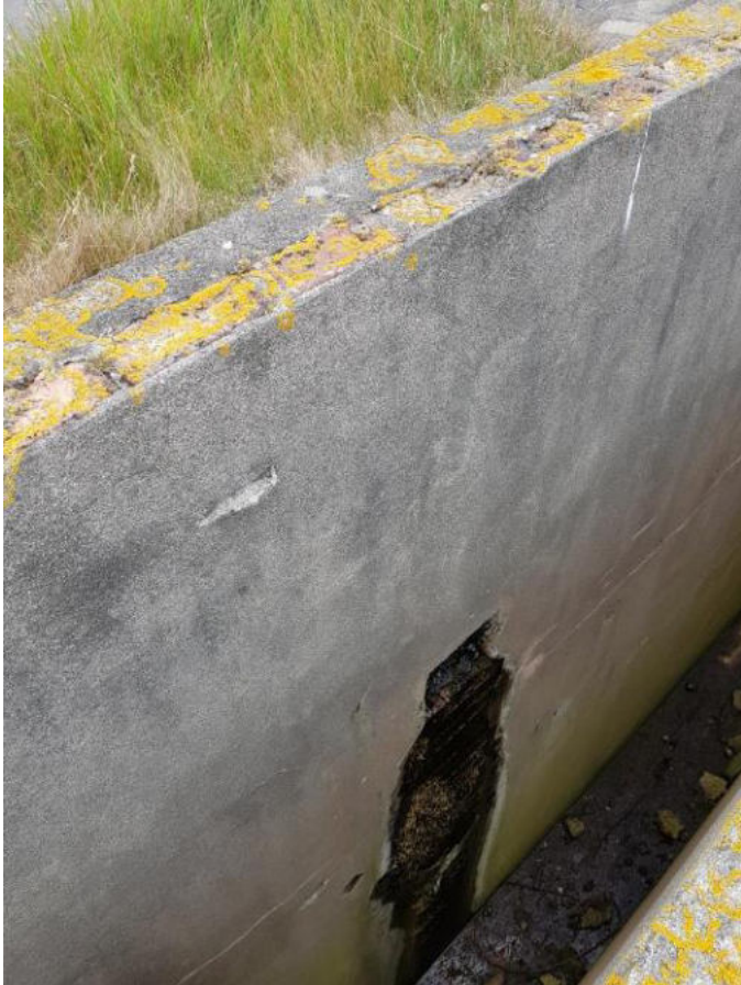
The outlet from the roof runs down into the wall and discharges part-way up it. Outlet is blocked by vegetation. Not loss of render from below the discharge point.
