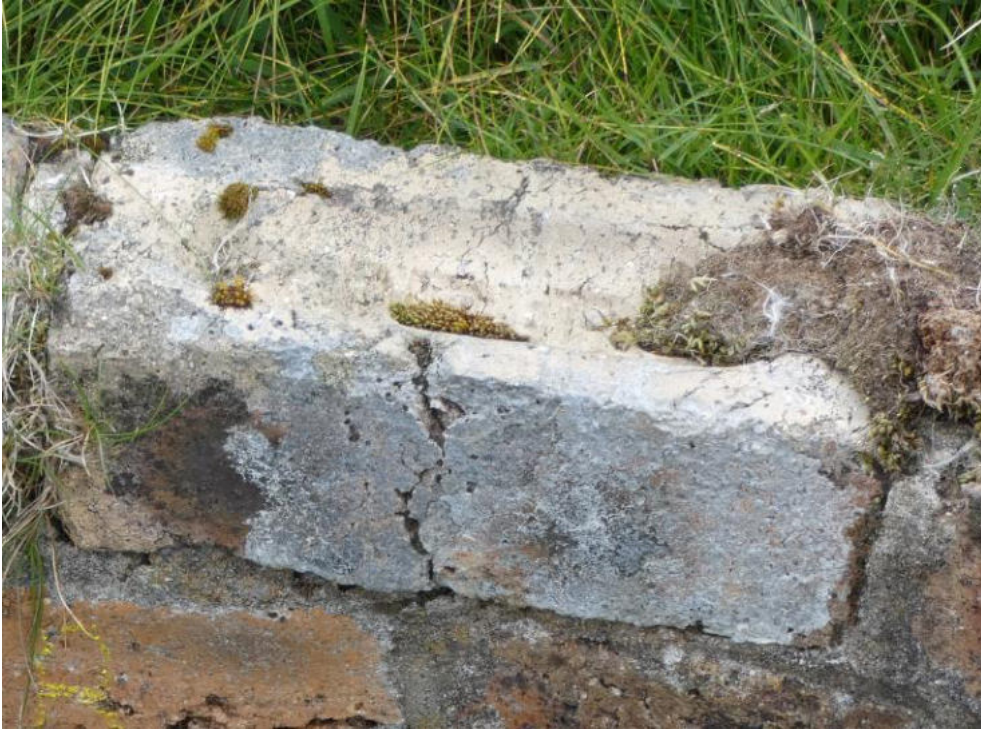
Localised failing joints at curved wallhead.
