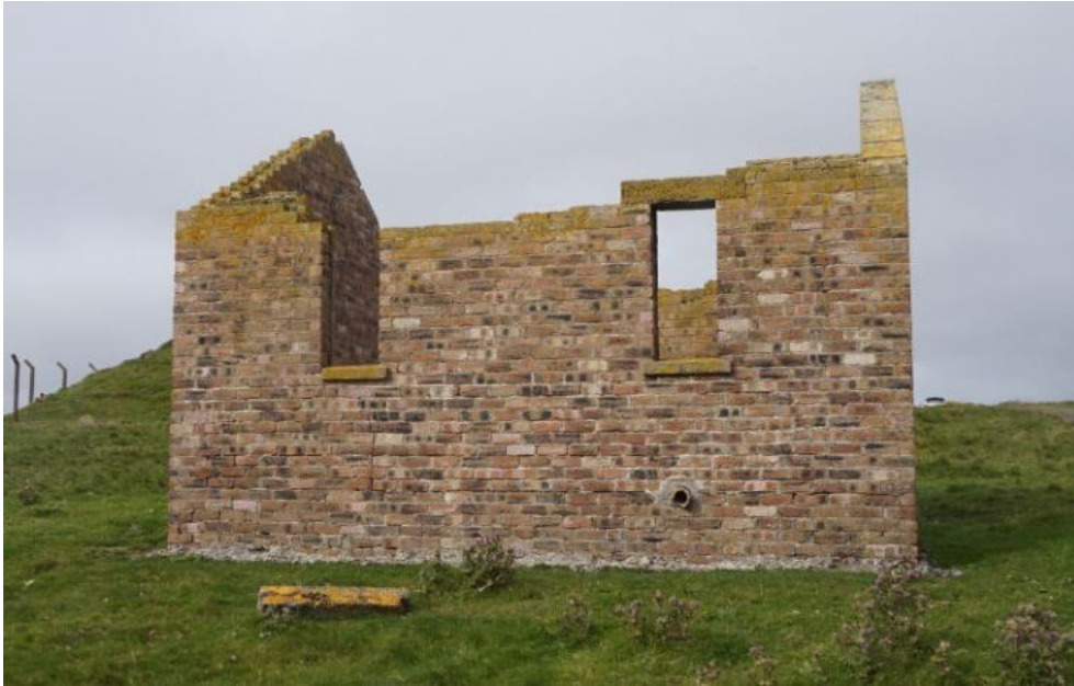
East elevation with dislodged lintel and fallen wallhead brickwork. To prevent ingress into the cavity, consider resetting the lintel and brickwork to allow the wallhead to be capped in concrete.
