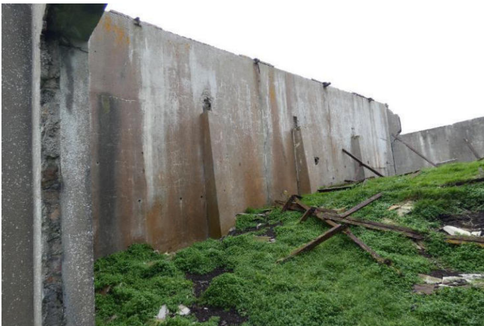
The internal piers do not appear to be fully or properly bonded to the masonry of the external walls.
