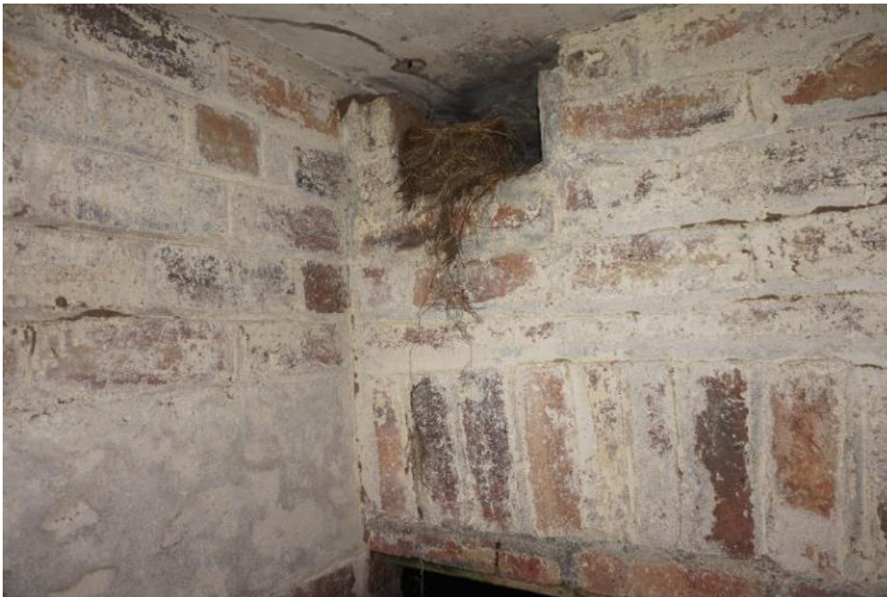
Nesting birds are using the structure.
