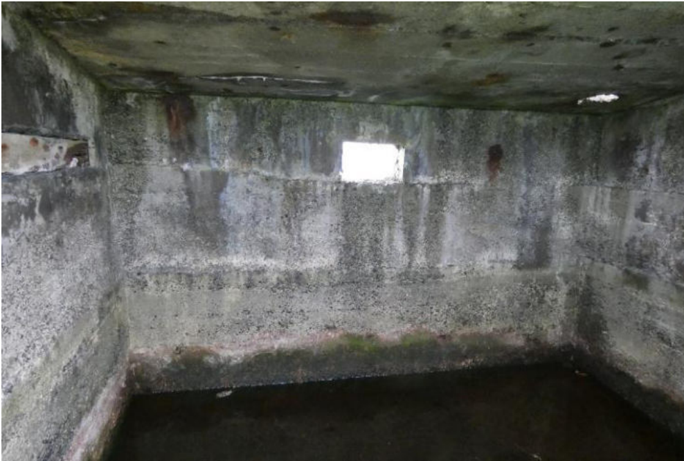
Hairline cracking, rust staining, leaching and discolouration to the walls exacerbated by flooding internally.
