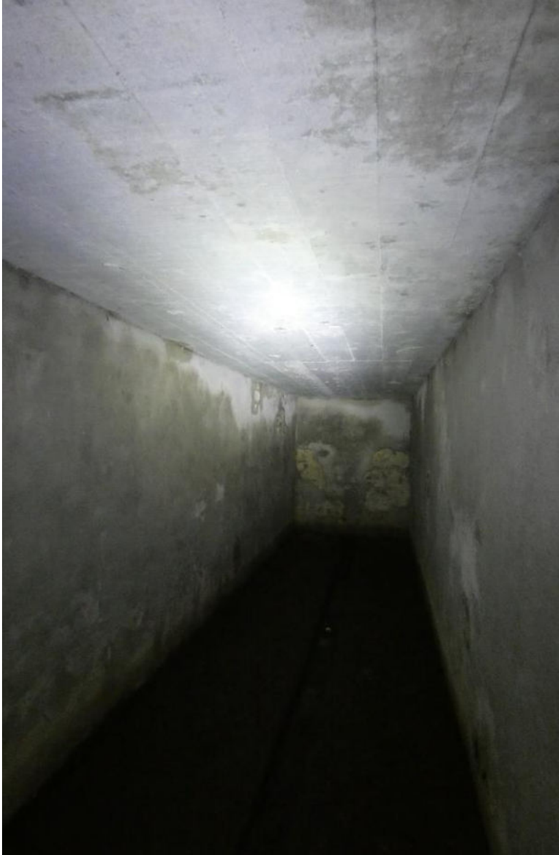
Localised failing render internally.
