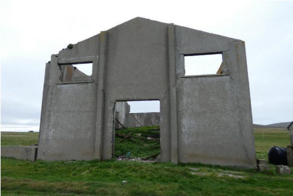
East elevation. Note the vertical cracking at each corner. Note the diagonal cracking between the entrance opening and both window openings and how this cracking continues up to wallhead: this elevation is a stack of independent, thin, tall, wall panels sitting atop each other.
