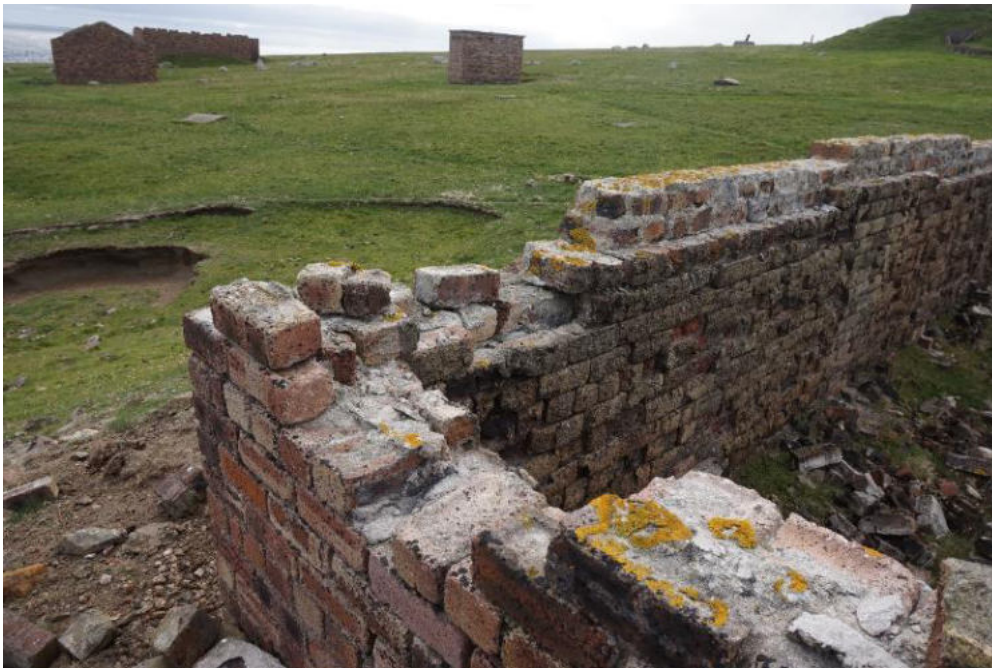
Loose wallhead brickwork and failing joints.
