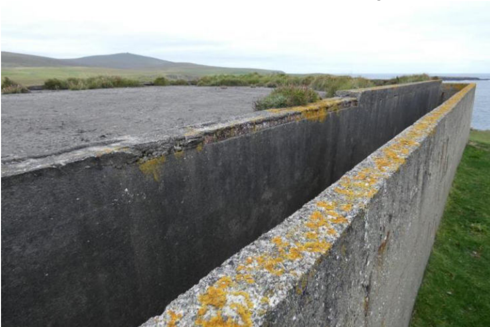
Looking across the surface of the roof. Note missing parapet copes and vegetation growing on roof.
