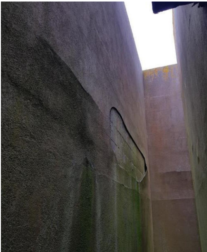
Note loss of render from face of blast wall.
