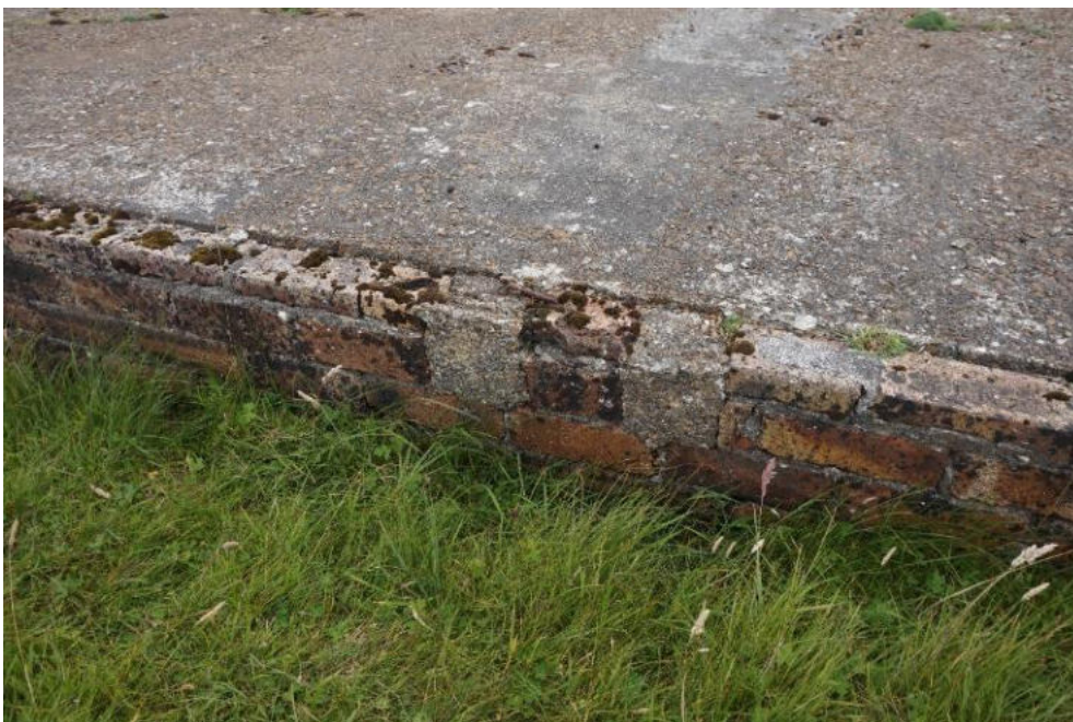
Stumps of reinforced concrete superstructure visible on the footings of the north and south elevations. Note cracked and failing mortar joints.
