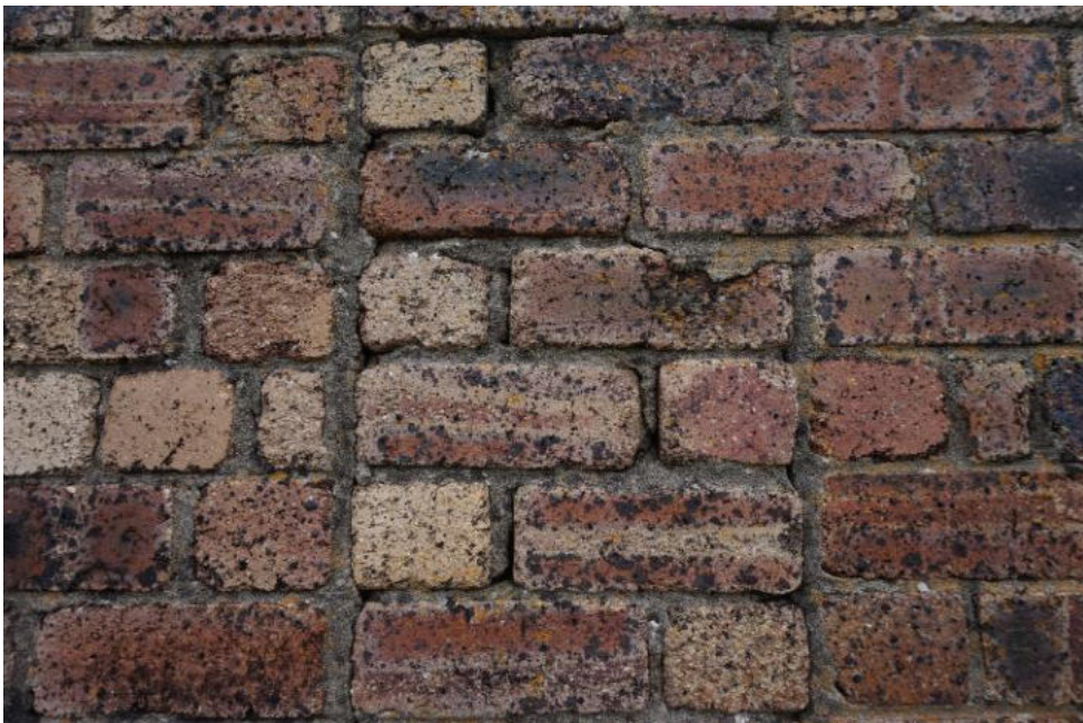
Localised failing wall face joints and minor cracking should be repointed. Note poor continuity between pier (middle of photo) and adjacent panels – see also photos 5 and 6.
