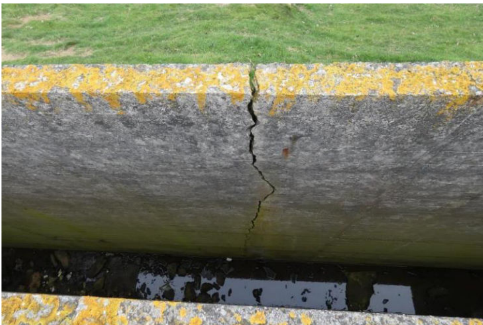
Vertical cracks in the blast walls are wider at the top of the wall than the bottom, indicating foundation movement. the provision of horizontal reinforcing bars appeared to be small.
