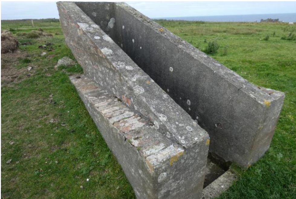
There is only minor damage to the rendered brick tunnel entrance.
