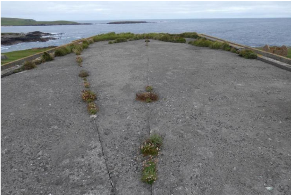
General view across the roof. Note cracking of the asphalt and vegetation growing from those cracks.
