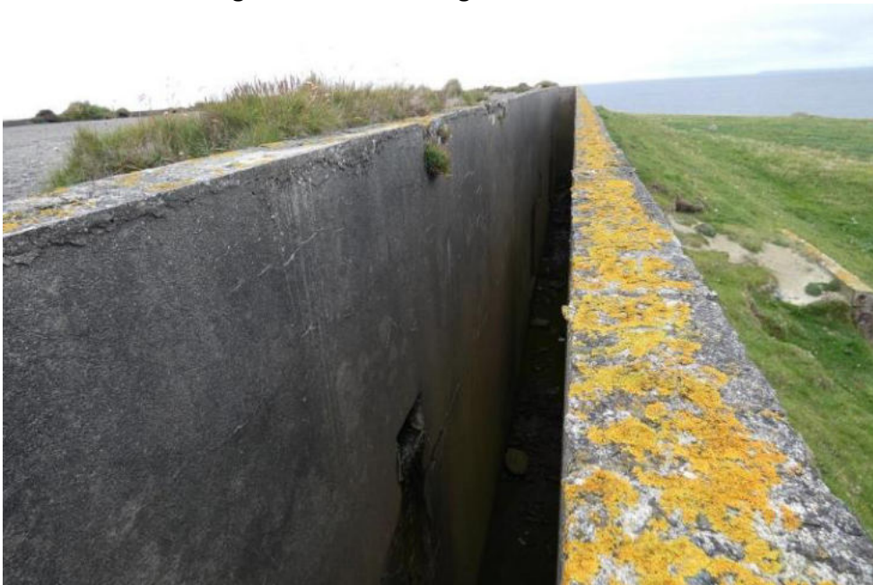
From the top of the embankment looking down into the gap between blast wall and building. The discharge point from the rainwater roof outlet can be seen partway down the wall of the building. vegetation growing from this outlet is blocking it.
