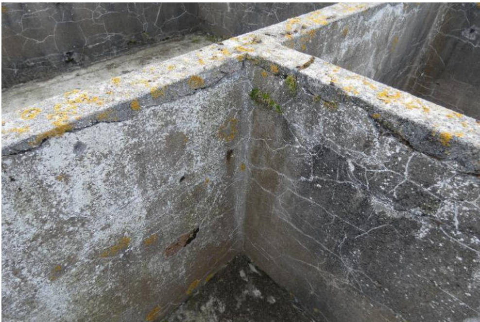
The render was patch repaired when the walls were lowered. All render (original and later) has cracked.
