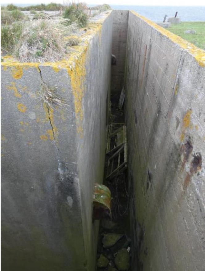
Note the debris across the floor of the perimeter lightwell. Note crack in the render of the building.
