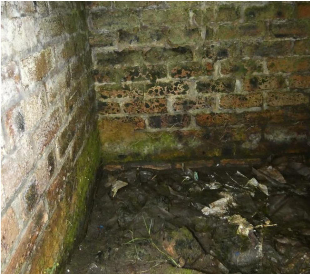
Saturated brickwork below covered area.
