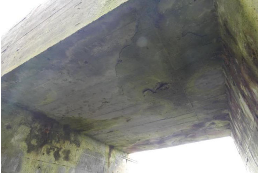
Spalling concrete and render finishes from the soffit of an access tunnel roof.
