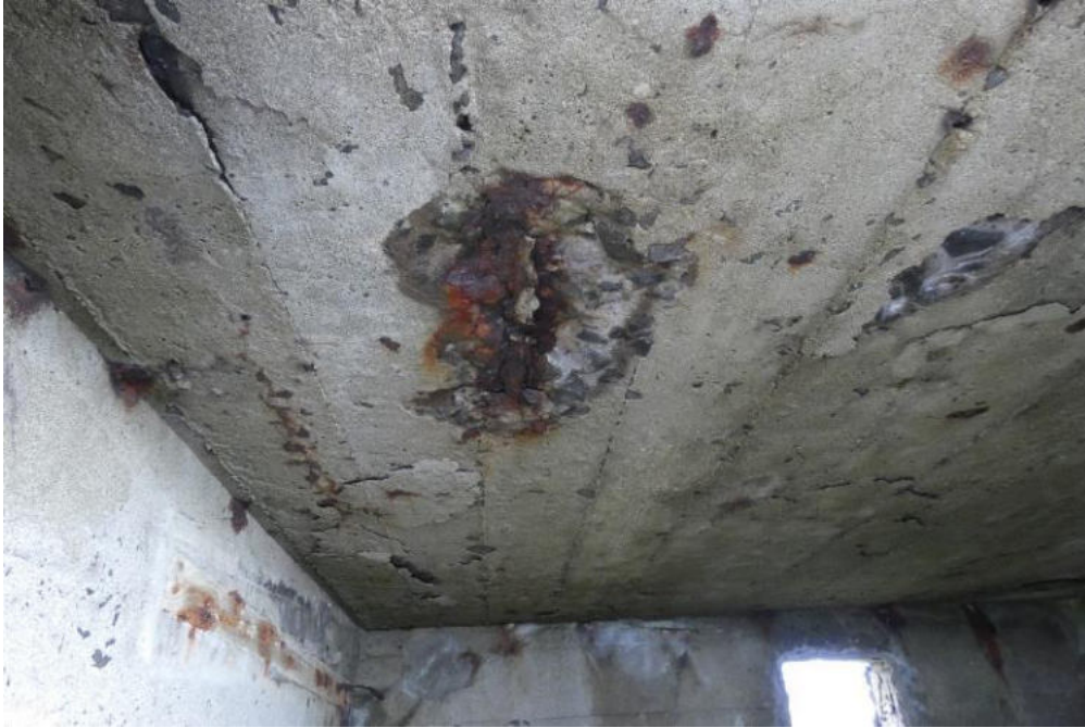
Localised spalling internally exposing corroded reinforcement.
