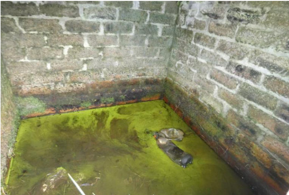
Flooded covered area saturating brickwork above.
