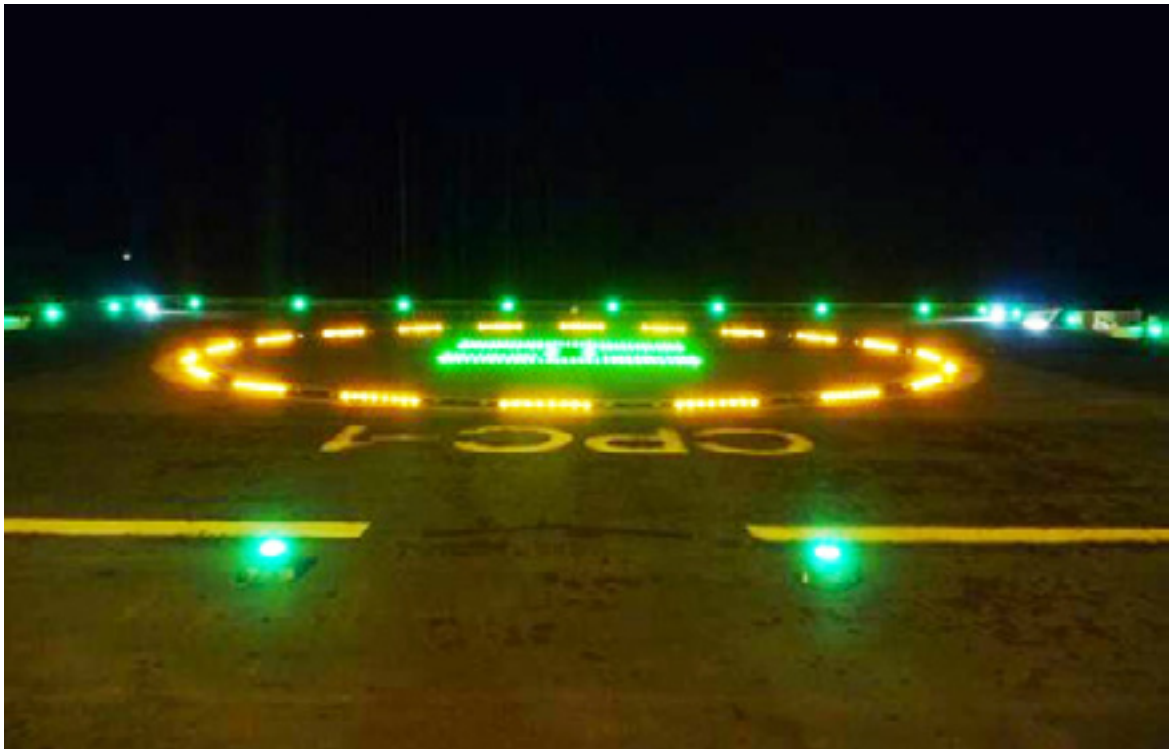
Figure 26 Orga by production lighting system on the CPC-1
