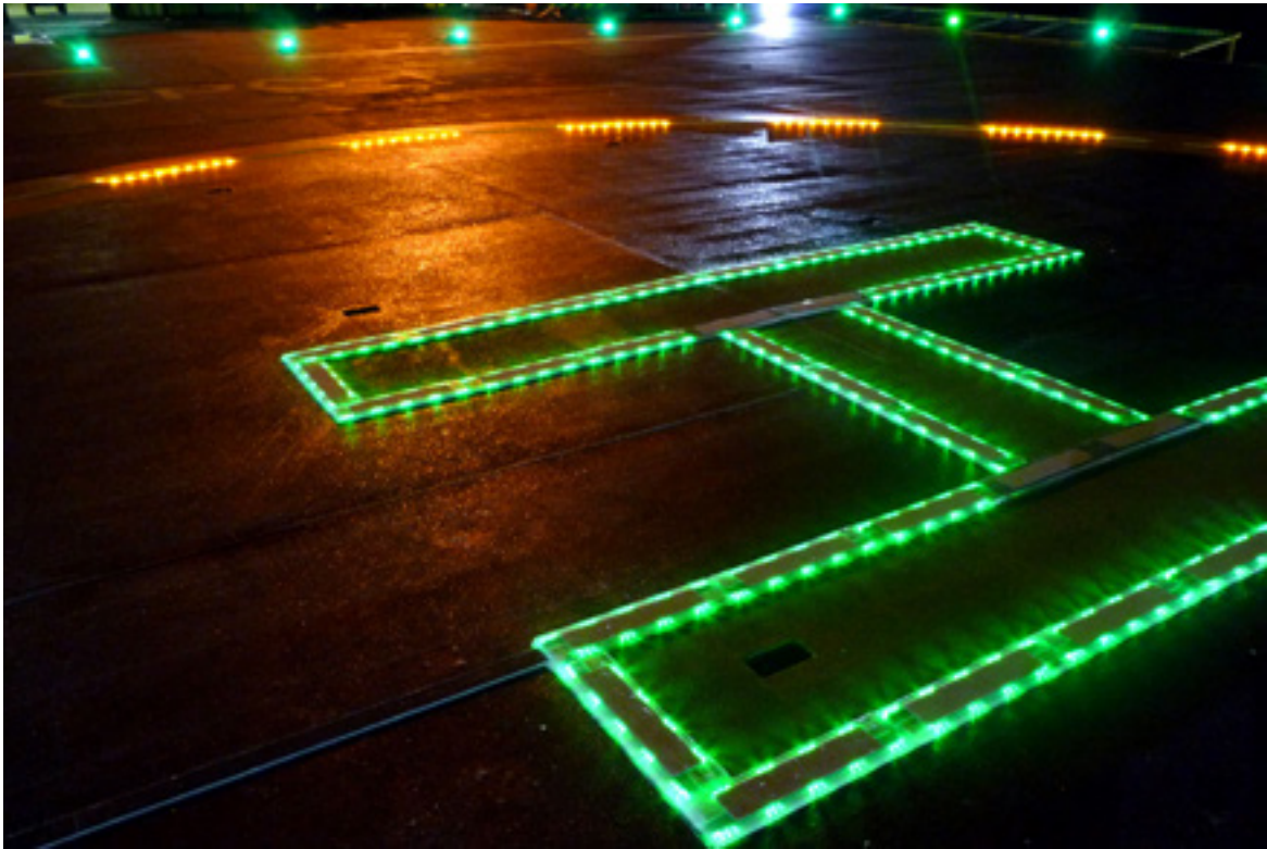
Figure 14 Heliport Identification Marking ('H') on the CPC-1
