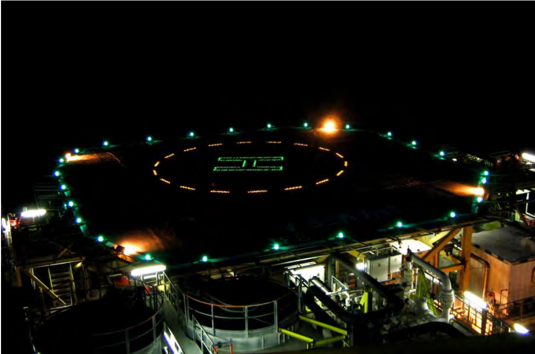
Figure 9 AGI prototype lighting system on the Thames A
