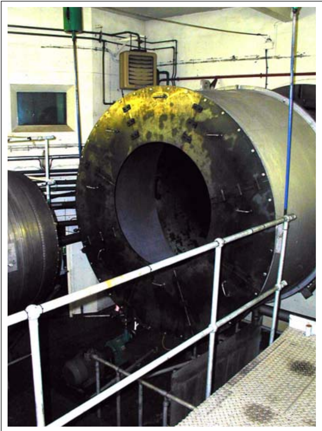
Figure 1 Detuner blocking plates (exhaust nozzle of the Spey Mk. 202 engine can be seen on the left)
