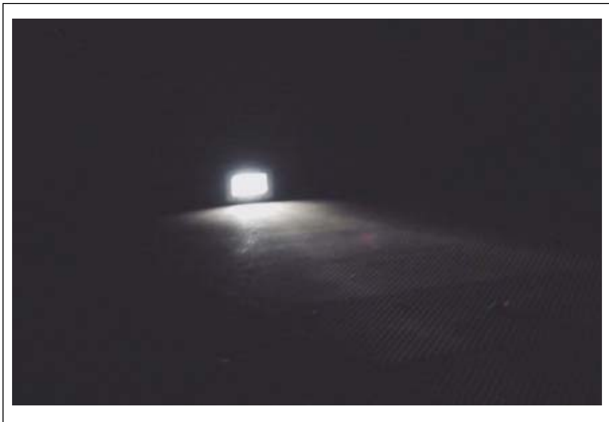
Figure 15 Floodlight Without a Hood
