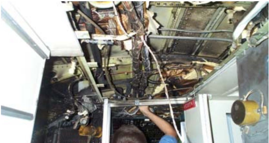
Figure 2 Fire in Bulkhead, Spread to Area Above Cabin Ceiling (Overhead)
